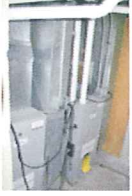
908 Midland Furnace Room.jpg
