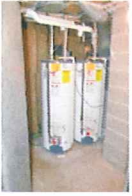
908 Midland Water Heaters.jpg
