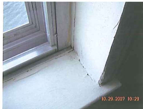
Existing interior window profile with typical adjacent jamb and sill deterioration
