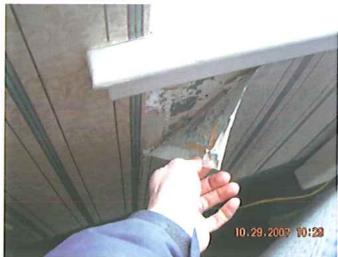
Existing damage at interior sills due to water migration through window frames
