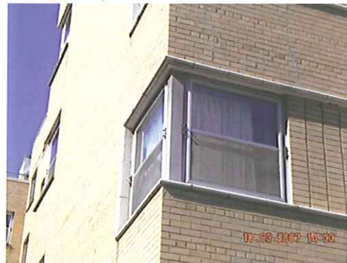
Existing exterior profile with pane divisions to be replicated in window systems replacement
