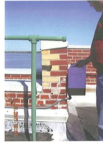
Example of parapet where masonry and roofing installation allow water penetration
