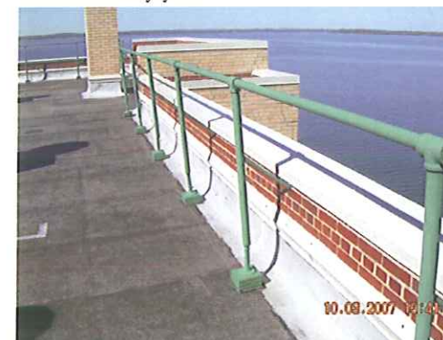
Existing roofing termination which promotes water infiltration into the exterior masonry system
