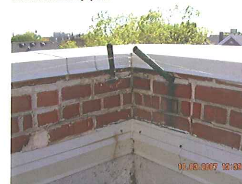
Existing roofing termination which promotes water infiltration into the exterior masonry system
