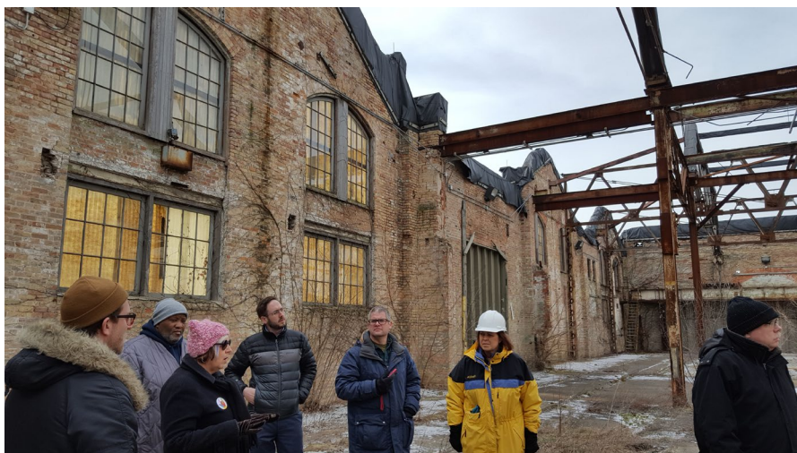
Figure 61: Landmarks Illinois board member Joshua Freedland (center), then with the design firm WJE, an Annual Corporate Sponsor, provides a pro bono condition assessment of the Rear Erecting Shops at Pullman National Monument, Chicago, Illinois, February 2017. Photo by Landmarks Illinois.
