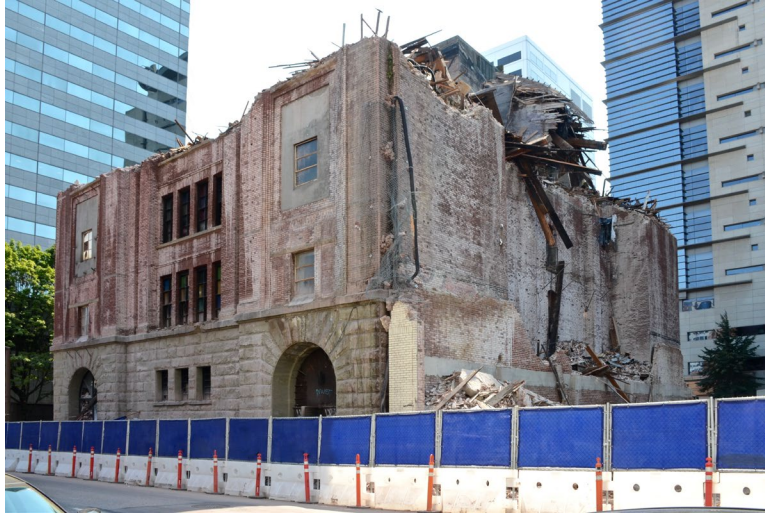
Figure 32: Demolition wastes reusable materials and generates carbon, such as this case with the destruction of Portland, Oregon's, Ancient Order of United Workmen Temple . Portland's groundbreaking deconstruction ordinance only applied to single-dwelling structures at the time. Not only were materials wasted, but also the opportunity to build proposed, needed affordable housing. Photo by Steve Morgan, September 3, 2017, CC BY-SA 4.0. Photo unchanged.
