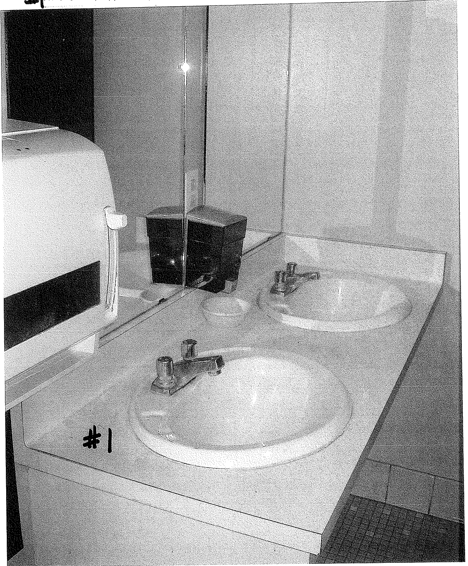
PHOTO # 2, MAIN TOILET - WOMEN #1 OUTDATED & NON-FUNCTIONING FIXTURES,
