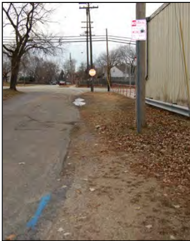
High Street looking west (poor condition)
