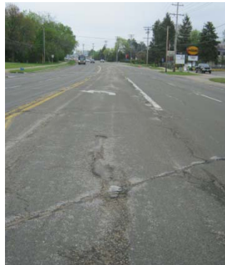
University Avenue, looking east (poor condition)
