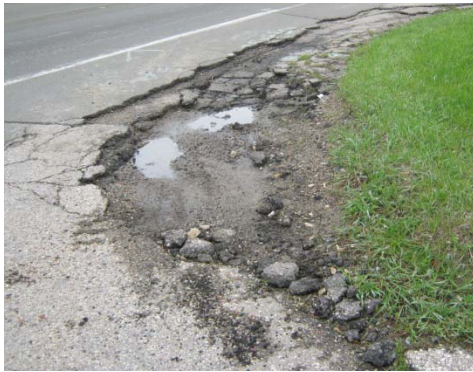
Asphalt problems along University Avenue (poor condition)
