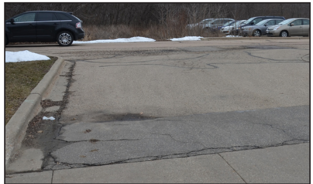
Pavement cracking, including patches; debris in gutter
