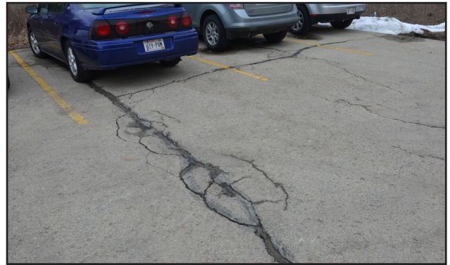
Pavement cracks and depressions
