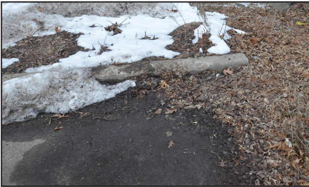
Corner of pavement covered in mud and debris, parking stop eroded
