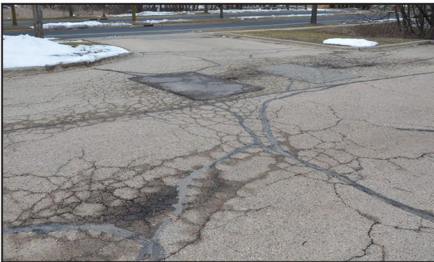
Pavement cracking, crumbling, including patched areas
