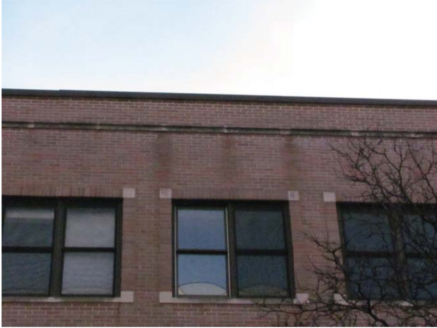
Figure 3. Water runoff staining below the stringcourse at the parapet wall.
