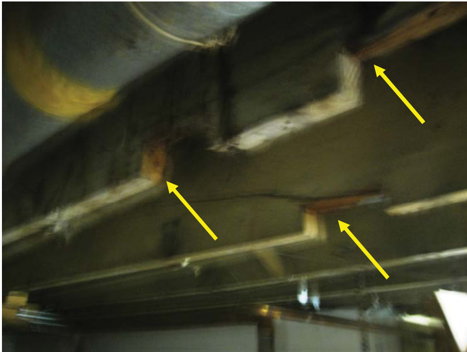
Photo 6 – Notched 1 st floor joists
