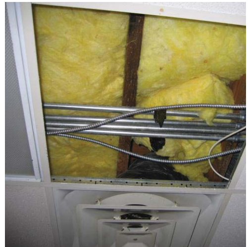
Conduits above ceiling on 3 rd floor.
