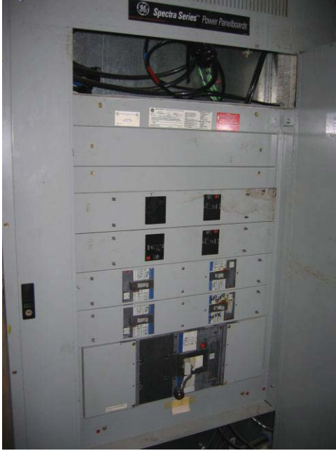
Distribution panel in the basement.
