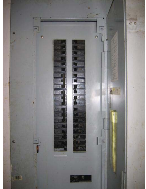
Electrical panel on 1 st floor restaurant.
