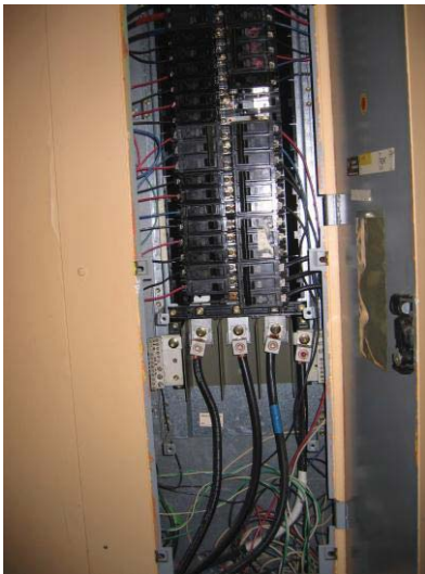
Electrical panel on 2 nd floor restaurant missing interior trim cover.
