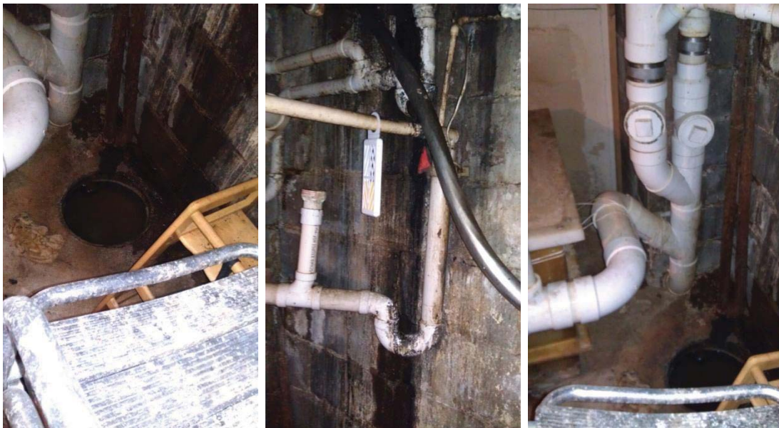
Poor condition of sanitary piping
