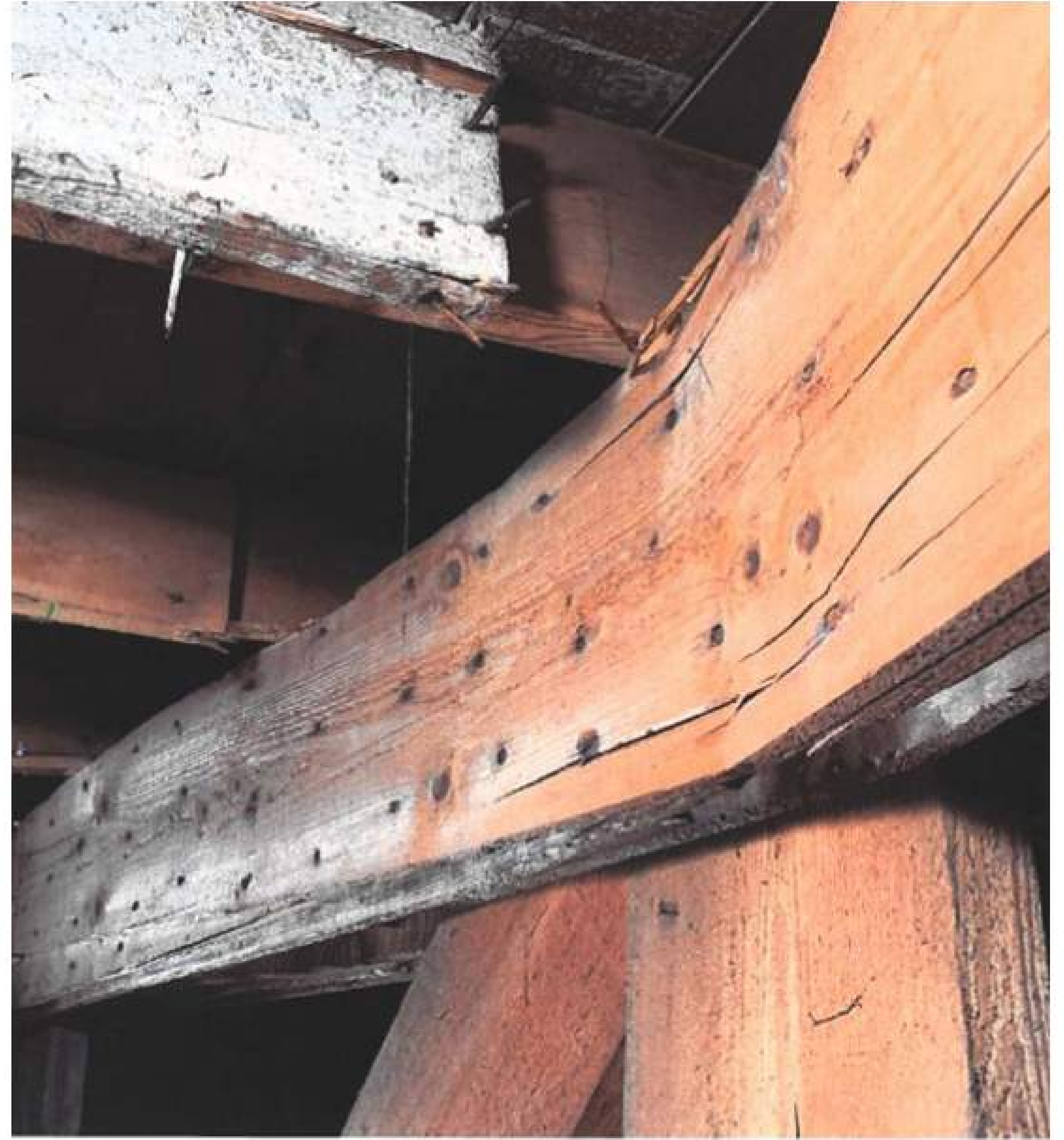
ROOF TRUSS & PURLIN FAILURE
