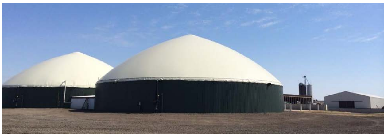
FIGURE 19: CYLINDRICAL DIGESTERS AT AGRIRENEW IN IOWA xxv
