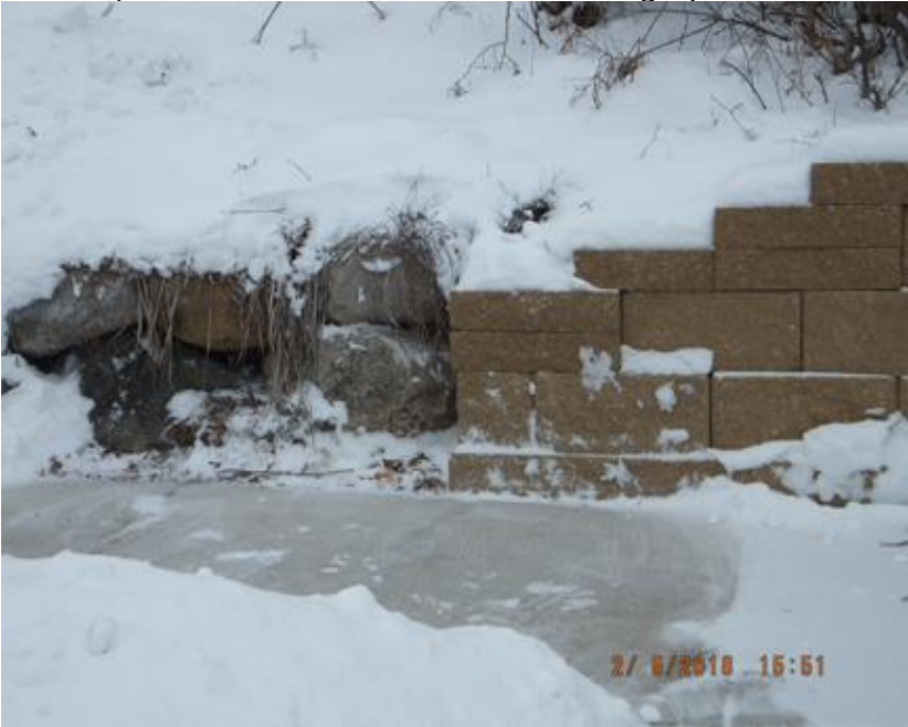
A new retaining wall, just wrapping the corner, could have met up with the boulder hillside at 520 Sheldon, as was done at this location on Gregory.
