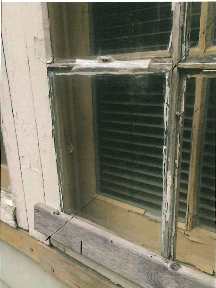
DETERIORATING GLAZING PUTTY
