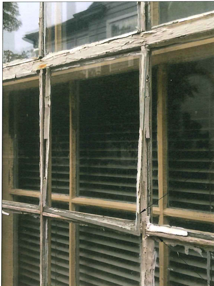
GLASS PANE FALLING OUT
