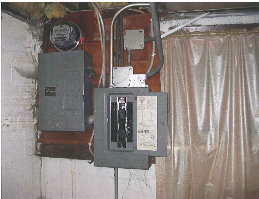
4817 Existing electrical service. Water damage observed on foundation wall
