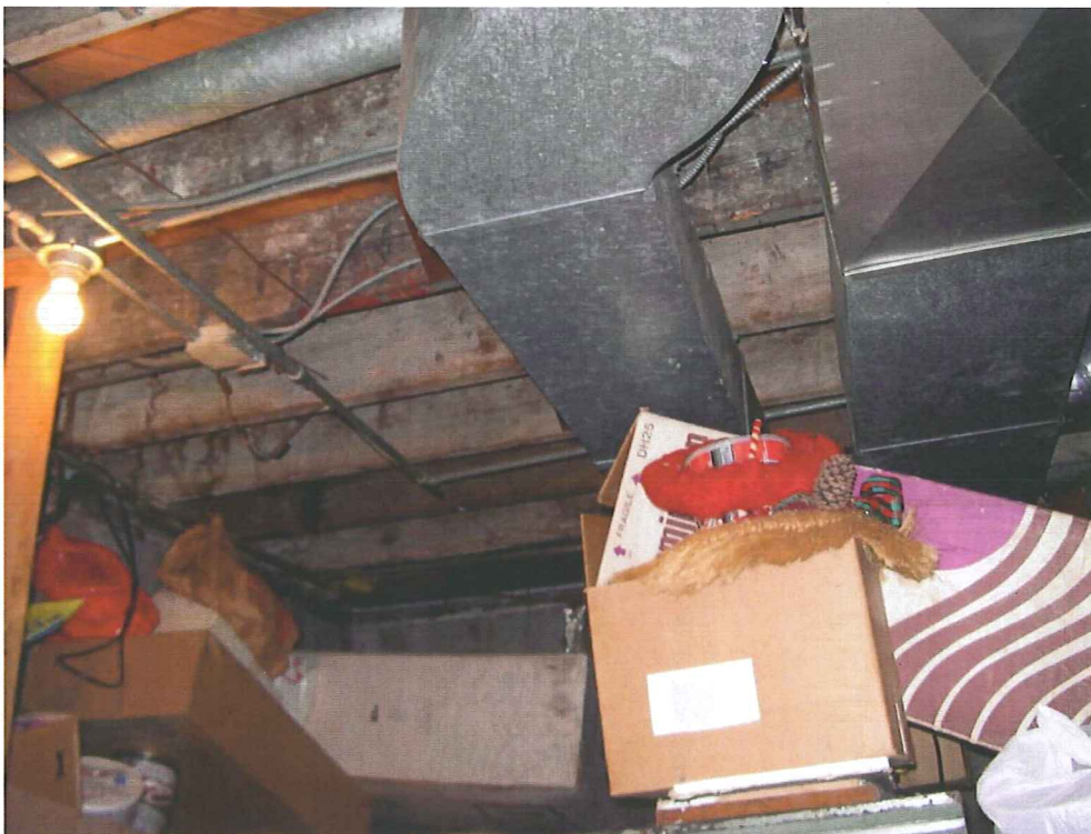
4817 Floor joist as visible from basement. Water damage was observed
