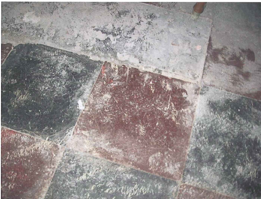
4817 Asbestos floor tile in basement
