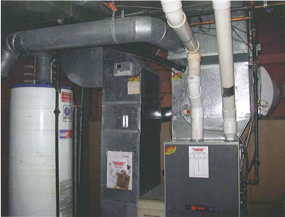
4817 Existing furnace and water heater
