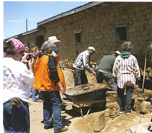
Restoration of the historic adobe stables at the Arkansas Valley Fairgrounds in Rocky Ford was a community effort. Volunteers learned how to make bricks and repair adobe structures, and various organizations came together to make the project a reality.
