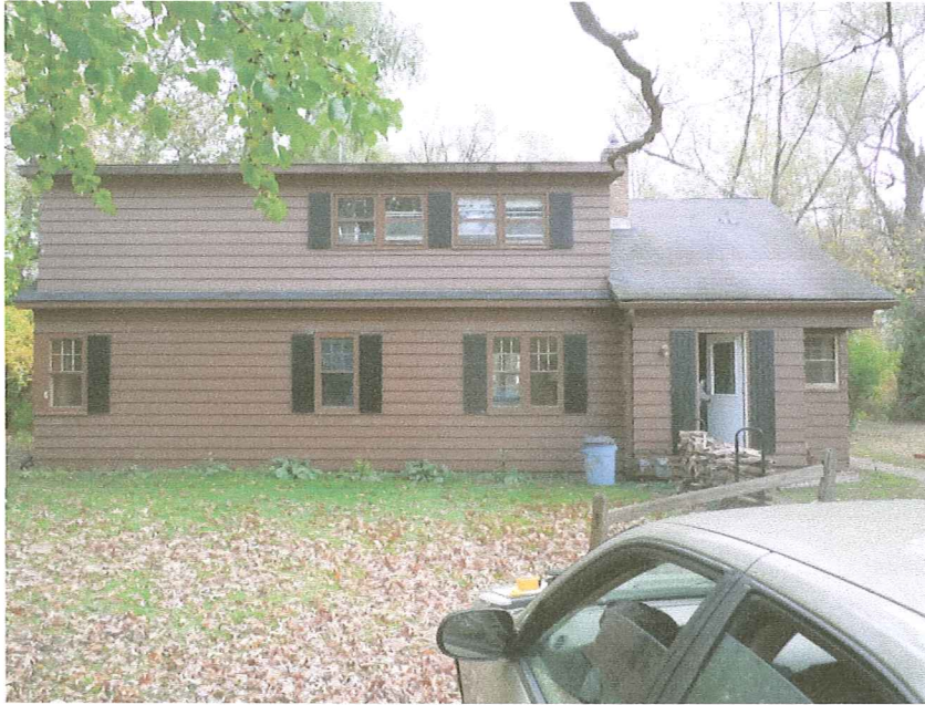
Lake Ripley House resting on a shallow foundation over a wet crawl space in a flood plain. Much of the framing of the first floor had rotted away.
