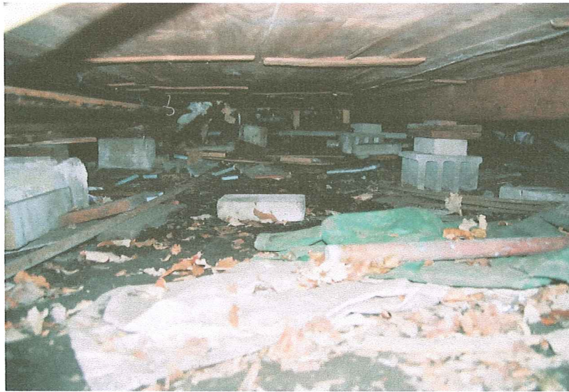
What passed for a foundation at 5980 Lake Edge, a collection of concrete blocks resting on wet soil. Note limited working room. Due to the soil and water table issues, a floating slab system was used to support the foundations. The framing was significantly twisted, but was not difficult to restore.
