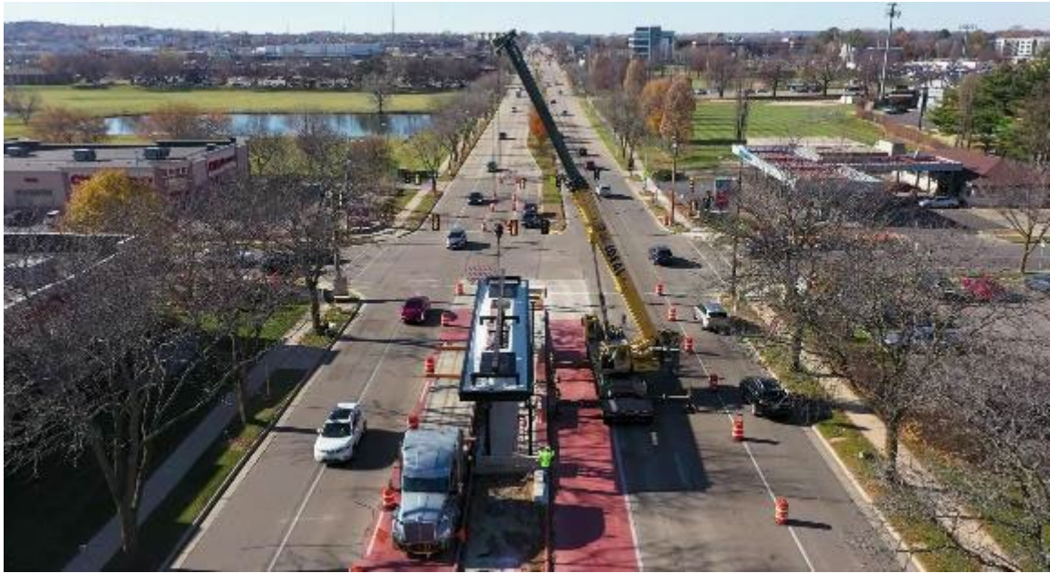
Figure 25 Erection of a Mineral Pt Rd BRT shelter. Photo courtesy of Wisconsin State Journal
