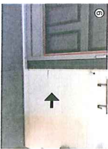
6 Replace cracked siding
