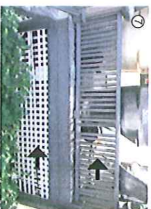
7 Replace deteriorated railing; replace lattice
