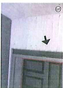
5 Replace cracked siding
