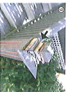
9 Repair/replace column trim
