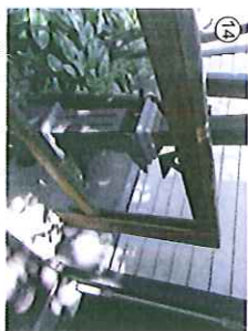
14 Repair/replace column trim
