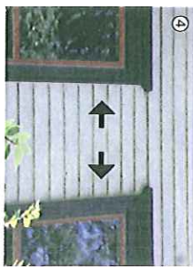
4 Replace cracked siding
