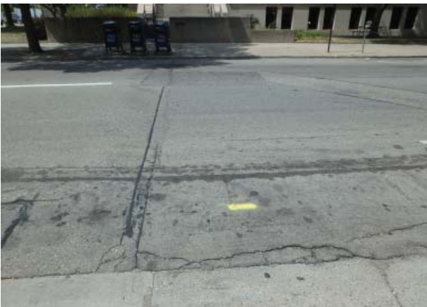
West Wilson near MLK Jr. Blvd (Fair condition)
