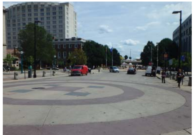
Martin Luther King Jr. Blvd (Good condition)
