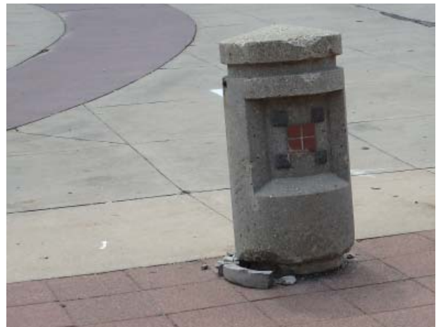
Martin Luther King Jr. Blvd Bollards (leaning & crumbling)
