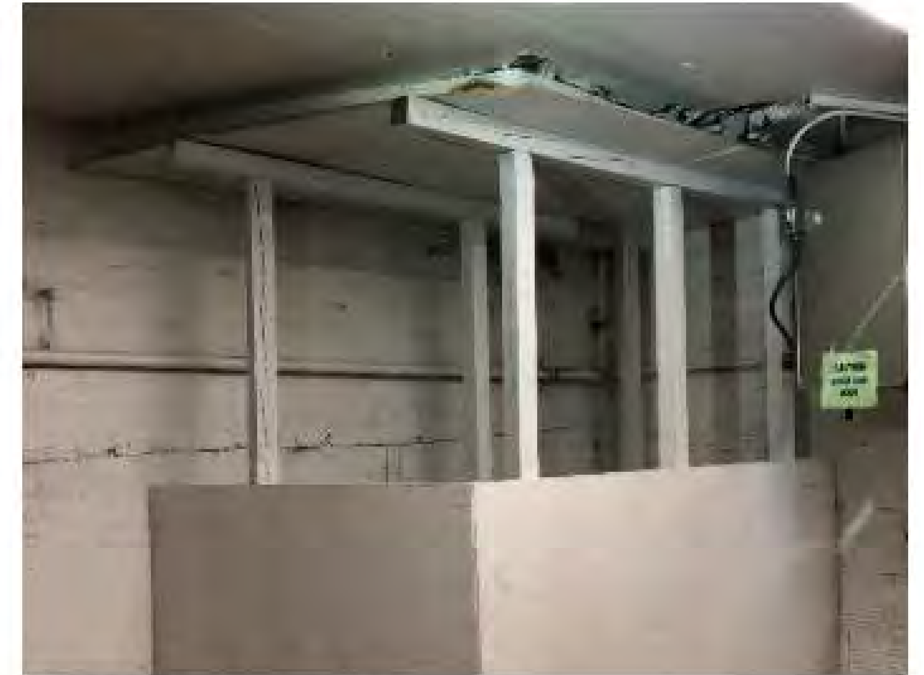
COLLAPSED FIRST FLOOR SLAB
