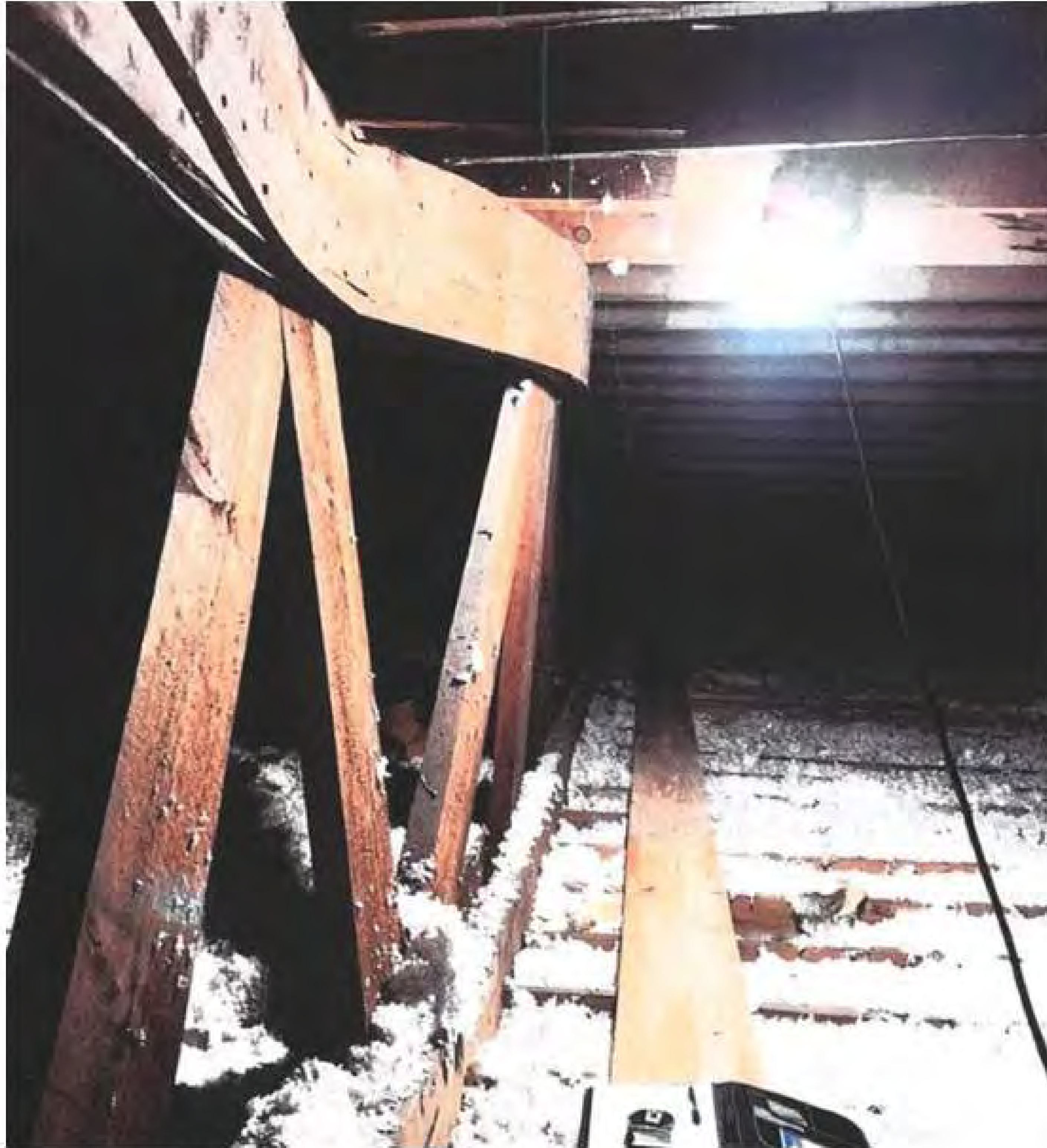
ROOF TRUSS FAILURE
