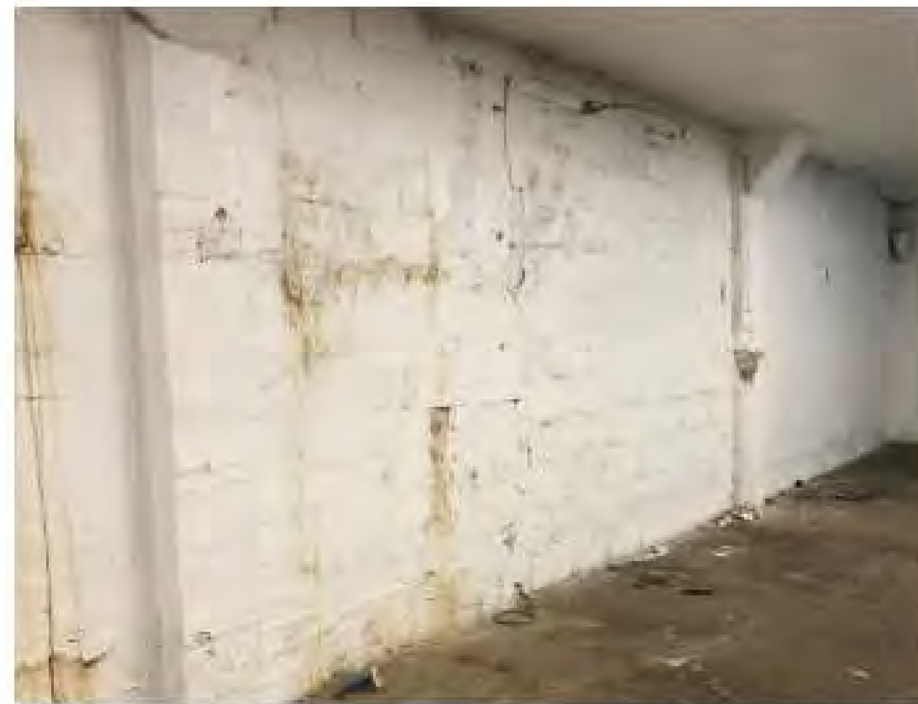
BASEMENT FOUNDATION WALLS DETERIORATED
