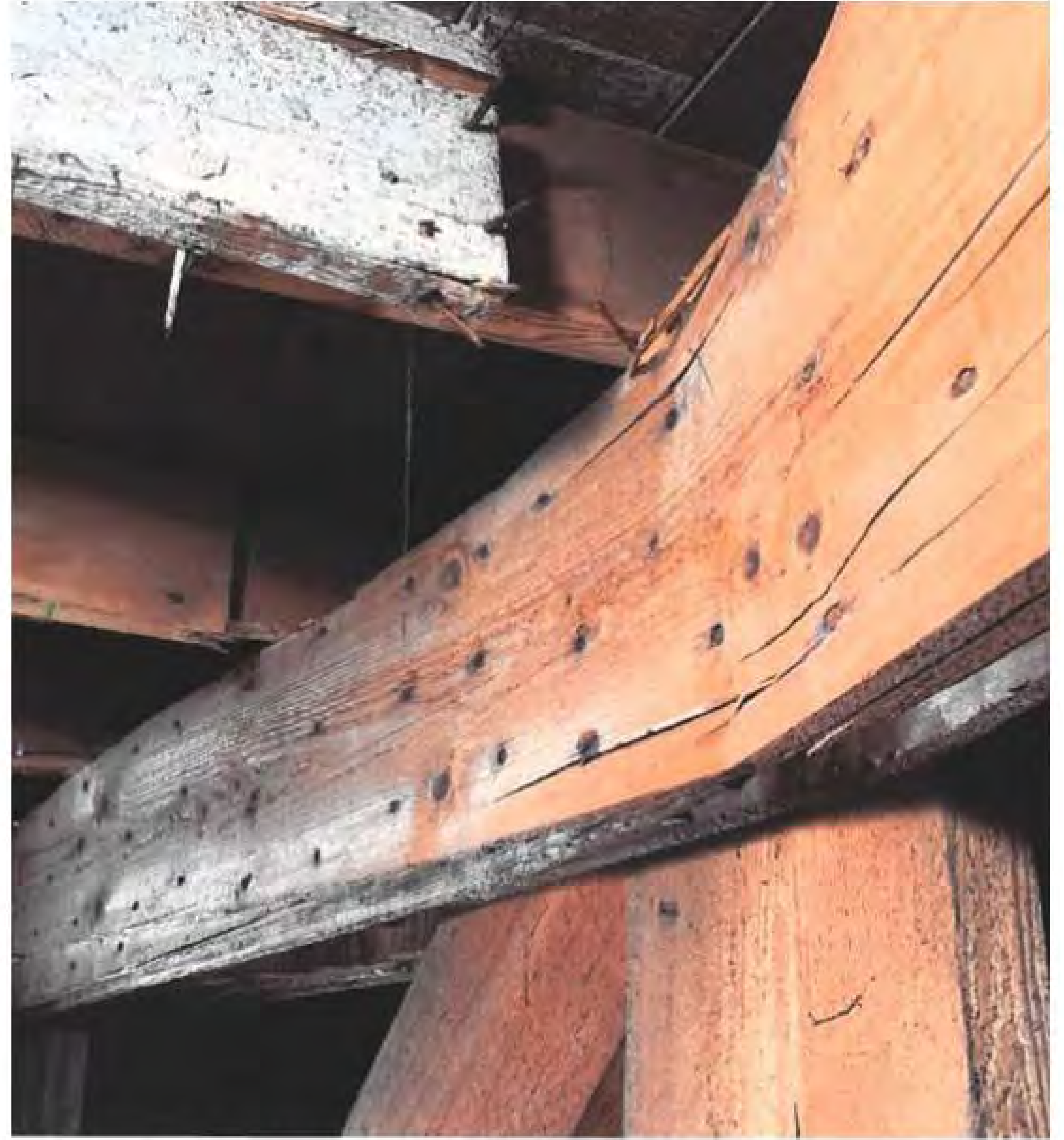
ROOF TRUSS & PURLIN FAILURE
