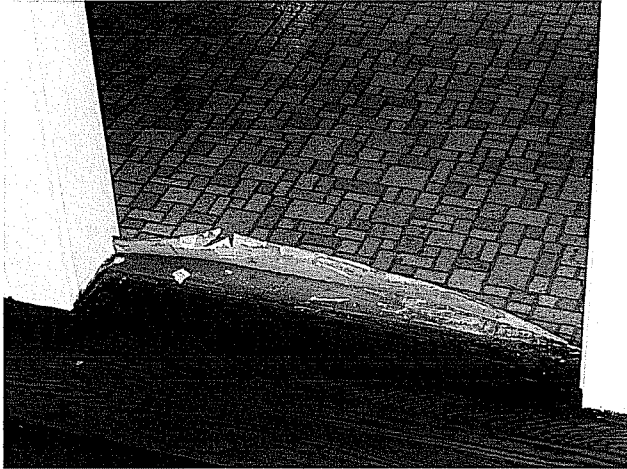
General state of disrepair
