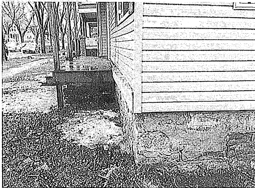
Image 6: First floor framing extending beyond the face of the foundation wall & exterior wall framing.
