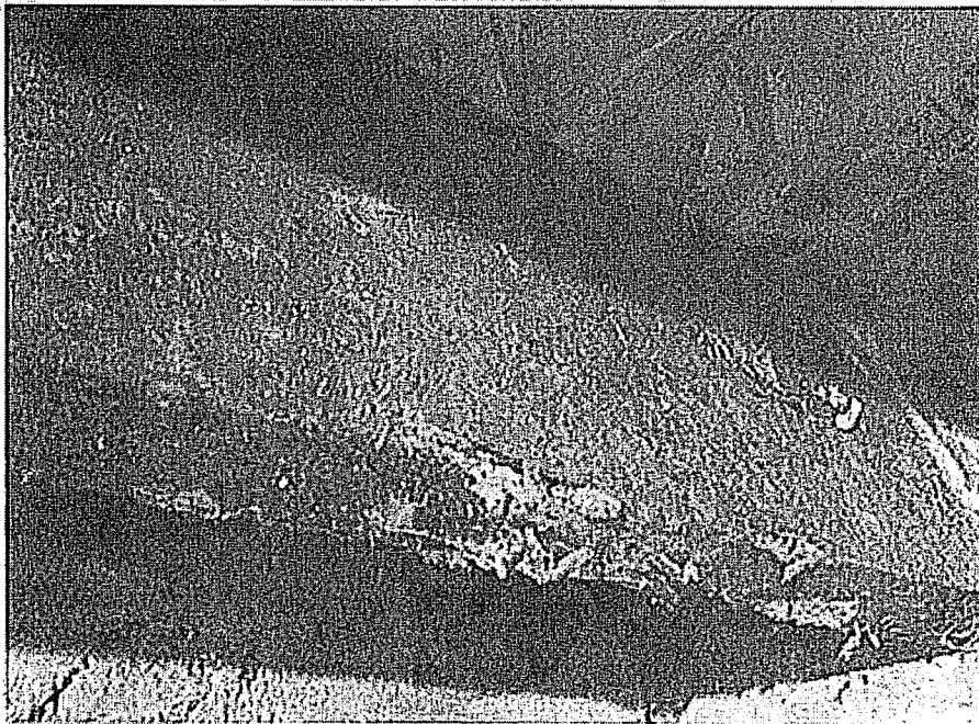
Image 26: Floor joist with apparent insect deterioration.
