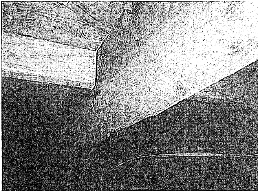
Image 30: View of damaged joist.
