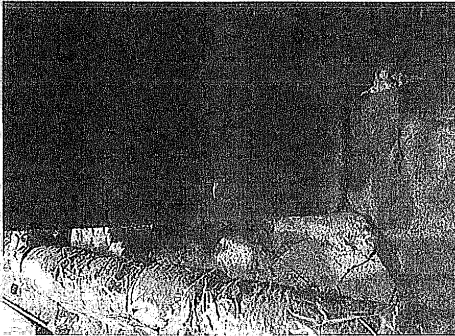
Image 11: Wood beam bearing directly on concrete with notch.
