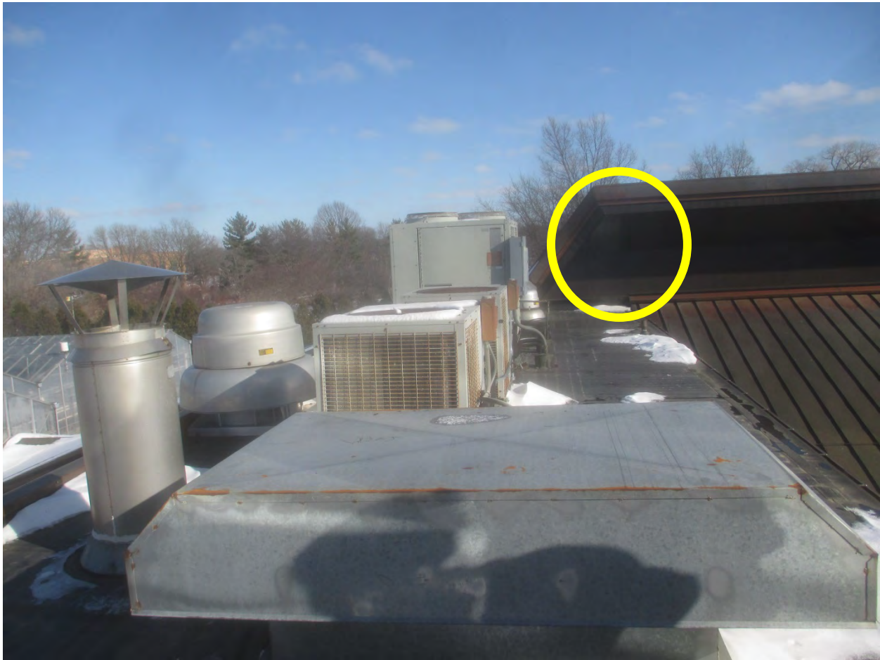
Figure 2 – Photo on flat roof area looking East. Note presence of roof top units but space is available to go above existing and future rooftop equipment if desired.
