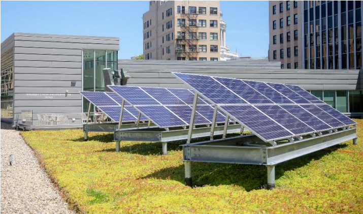
Solar Installations & Green Roofs
