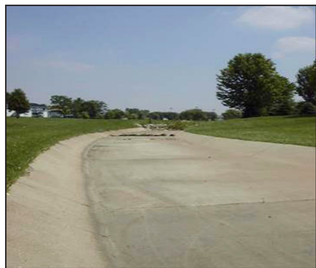
Figure 4 - Concrete drainage swale (an example of “grey” infrastructure) prevents rainwater infiltration and groundwater recharge. Orgeon, WI.
