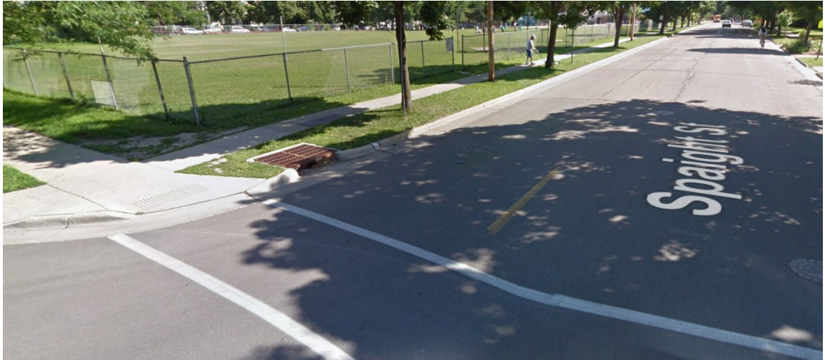
Figure 9. Terrace inlet at Spaight & Dickinson.
