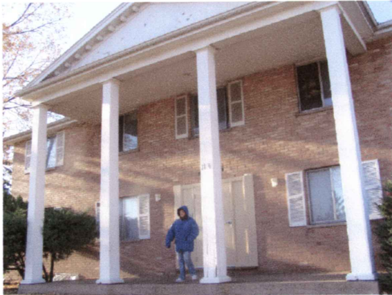
1114 Ann Street Deteriorated porch posts October 25, 2003
