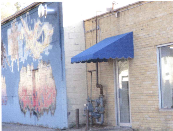
1817 South Park Street Cracked wall October 25, 2003
