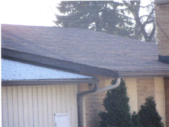
1823 South Park Street Deteriorated shingles and boarded windows October 25, 2003
