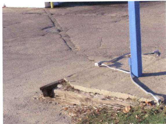
1824 South Park Street Deteriorated sign base October 25, 2003
