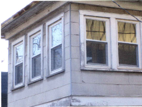
1810 Beld Street Deteriorated windows October 25, 2003
