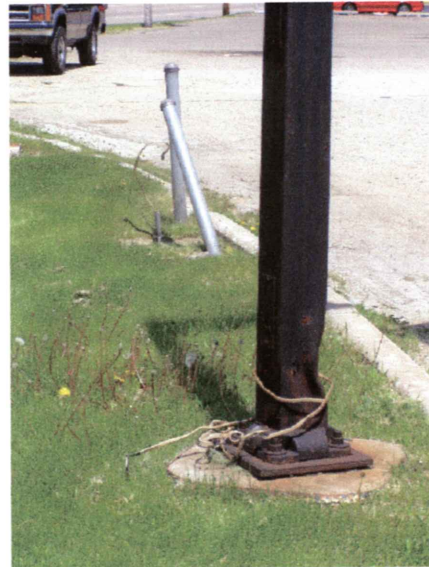
2421 South Park Street Exposed wiring, bent and dented posts May 25, 2003
