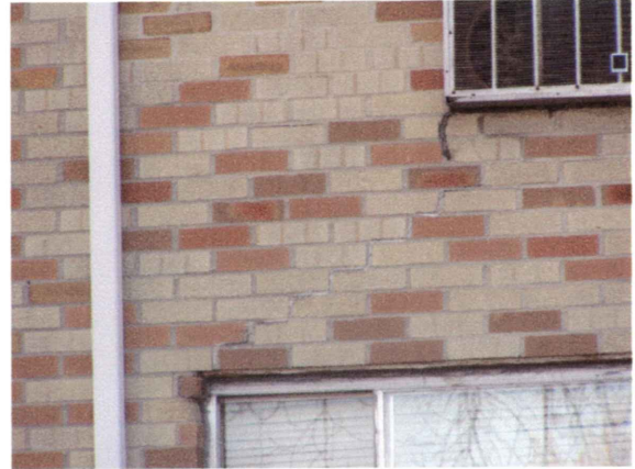
1114 Ann Street Cracked Wall October 25, 2003
