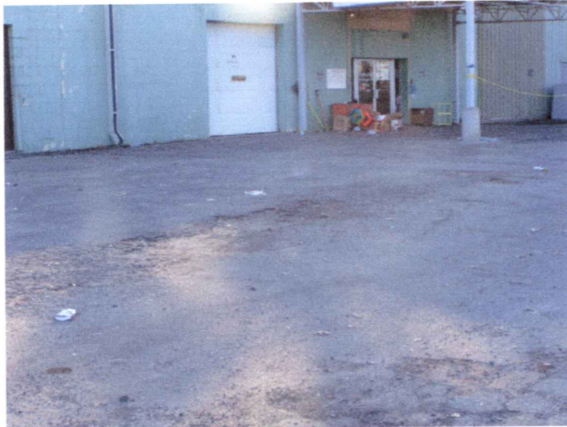
1500 South Park Street Deteriorated drive October 25, 2003
