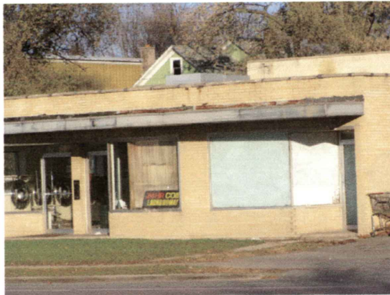
1817 South Park Street Deteriorated roof October 25, 2003
