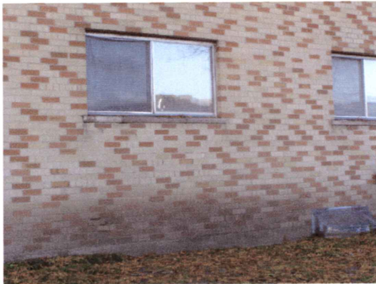
1114 Ann Street Water damaged wall October 25, 2003
