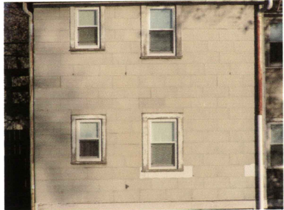
1810 Beld Street Deteriorated wall and window frames October 25, 2003
