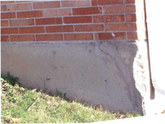
1114 Ann Street Cracked foundation October 25, 2003
