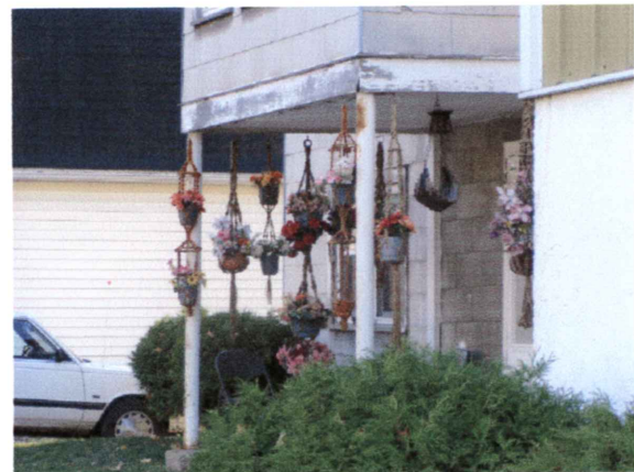
1810 Beld Street Rotted porch October 25, 2003
