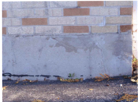
1114 Ann Street Cracked foundation October 25, 2003
