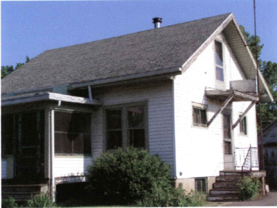
836 Hughes Place Deteriorated porches and roof at May 25, 2003
