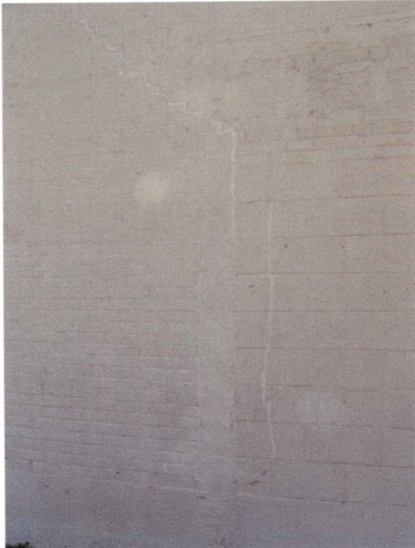
1818 South Park St Cracked Wall October 25, 2003
