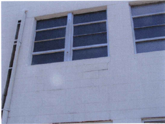
2216 South Park Street Cracked Wall May 25, 2003
