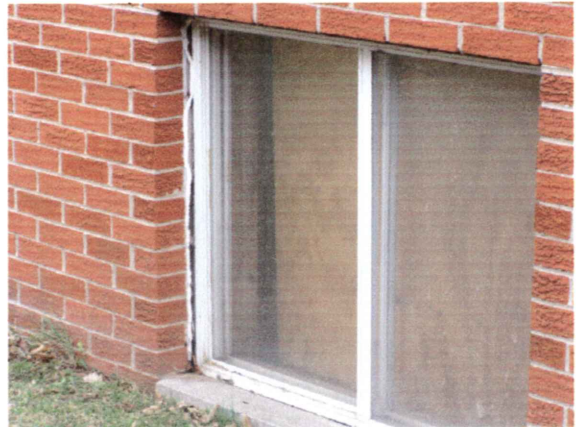
2306 Badger Parkway Deteriorated window frame October 25, 2003
