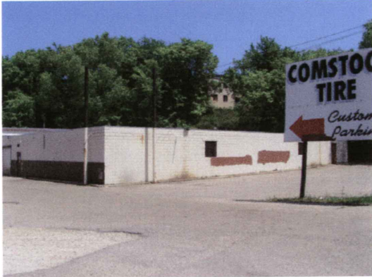
2421 South Park Street Blighted driveway and parking lot, water damaged wall May 25, 2003
