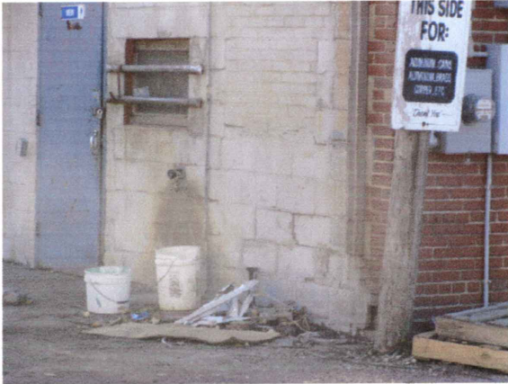
1818 South Park Street Trash and cracked wall, deteriorated door and window October 25, 2003
