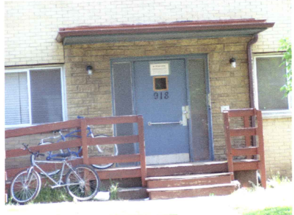
918 Magnolia Lane Deteriorated porch, steps and unsafe steps May 25, 2003
