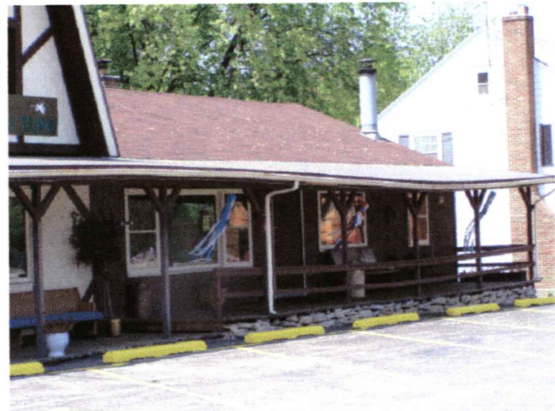
2465 South Perry Street Sagging Roof May 25, 2003
