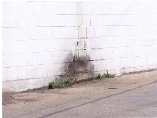
2431 South Park Street Cracked and water damaged wall, May 25, 2003
