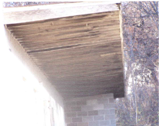
1818 South Park Street Rotten fascia and roof joists October 25, 2003
