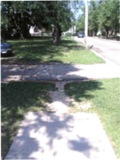
Badger road Missing Sidewalk July 7, 2005
