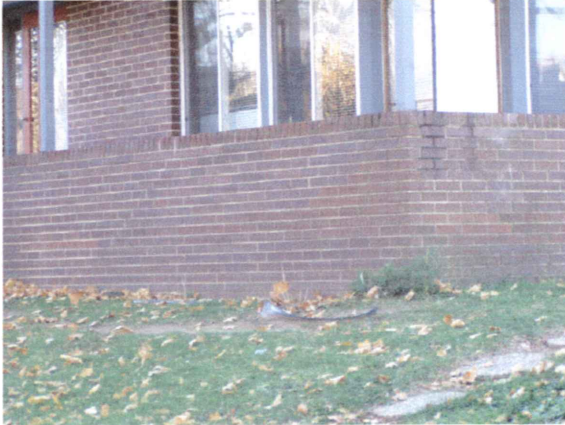
1850 Beld Street Cracked wall October 25, 2003
