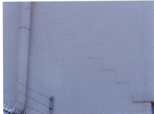
1818 South Park Street Cracked Wall October 25, 2003
