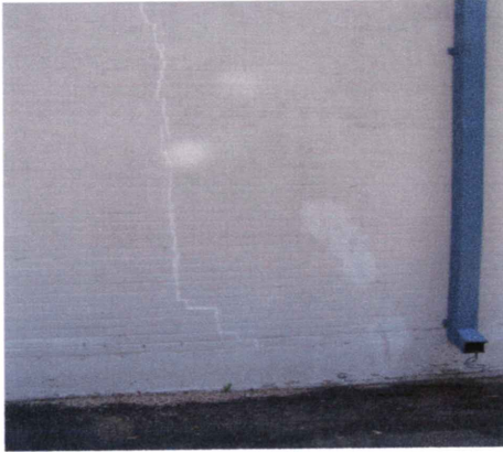
1818 South Park St Cracked Wall October 25, 2003
