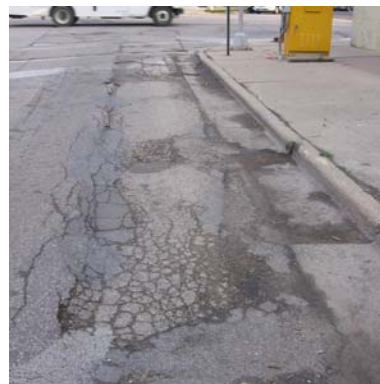
Butler and Johnson, looking northwest (patchwork, cracks, and missing asphalt)
