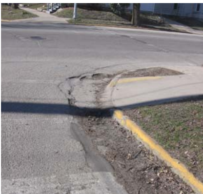
Franklin and Johnson, looking northwest (debris, patchwork, missing concrete/asphalt)
