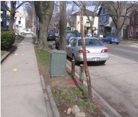
Johnson and Franklin, looking northwest (rusted pole support and bollards)
