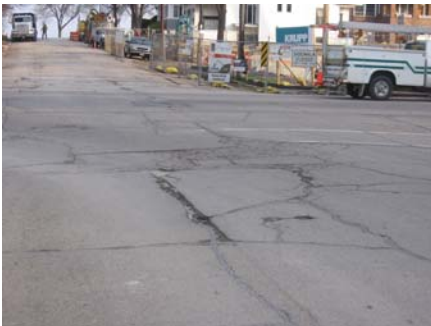
Blair and Johnson, looking northwest (cracks, patchwork, and missing asphalt)
