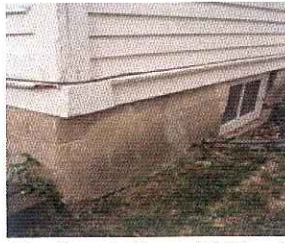
The foundations of 415 and 417 contain concrete block.
