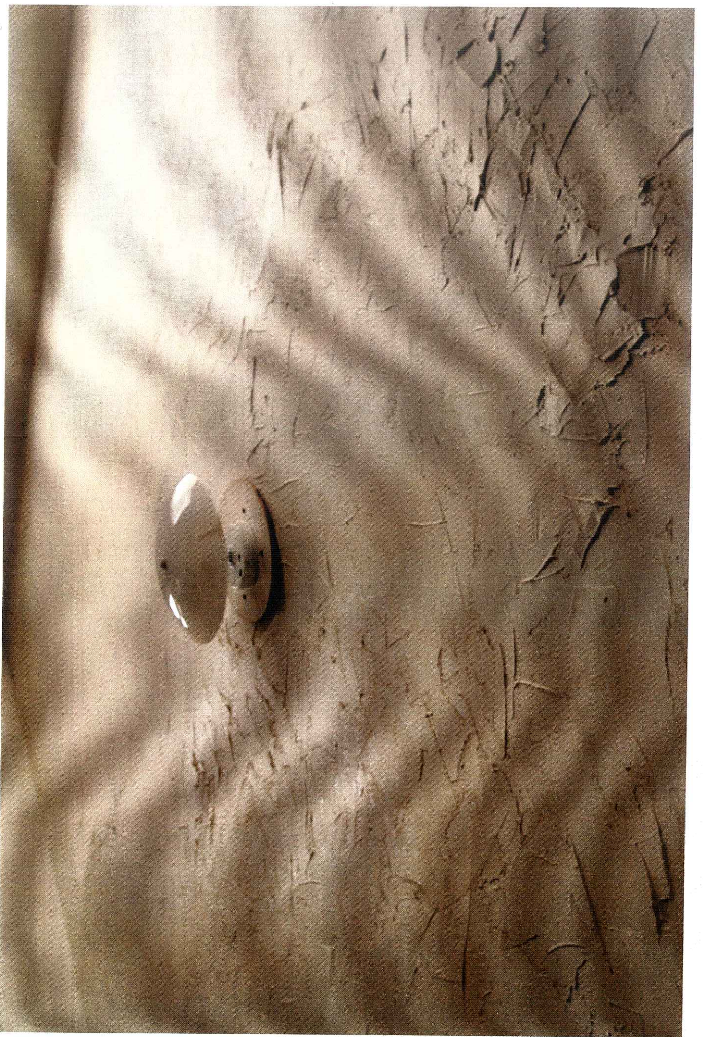
EXAMPLE OF FALLING LATHE AND PLASTER CEILINGS
