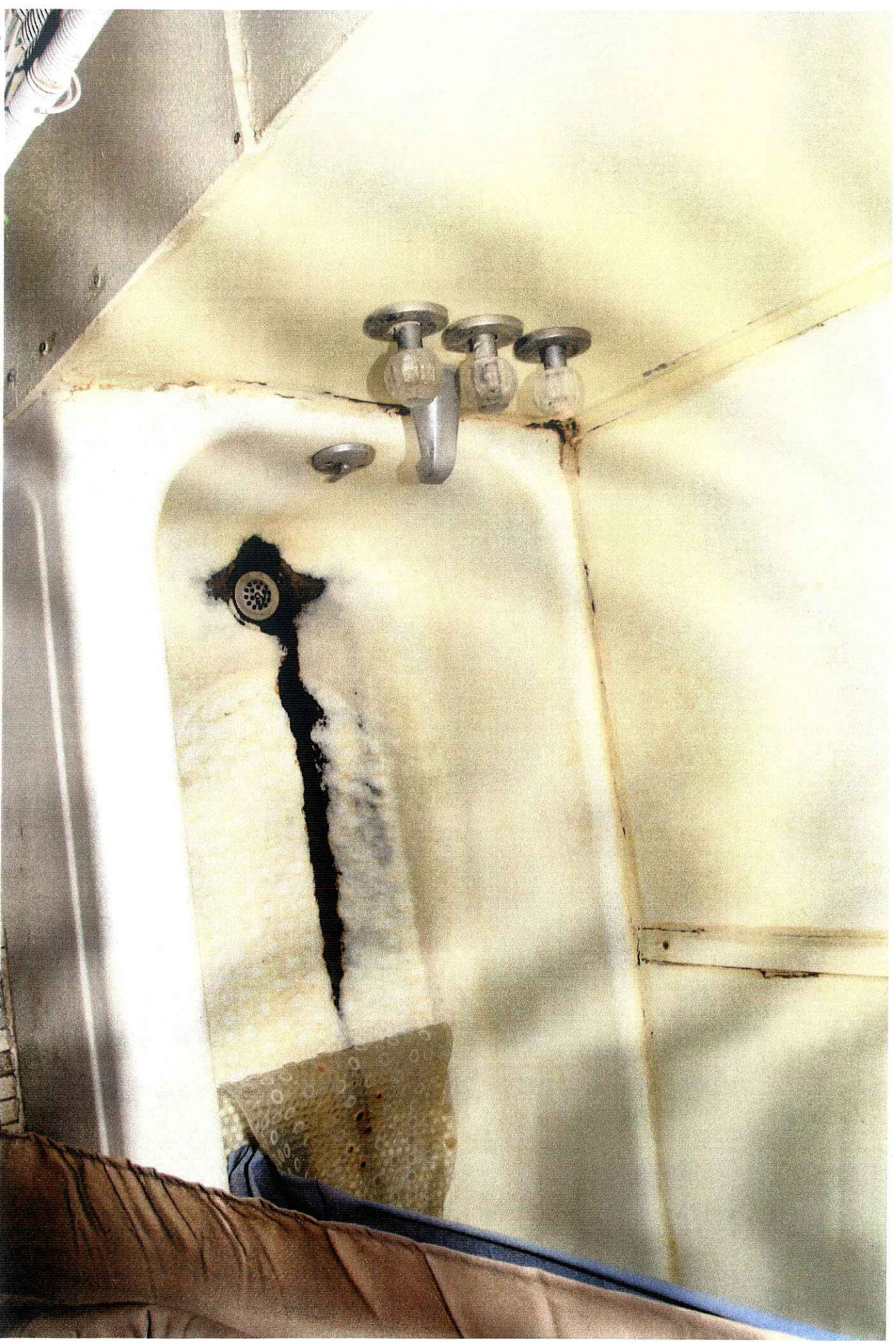
EXAMPLE OF WORN OUT BATHROOM FIXTURES
