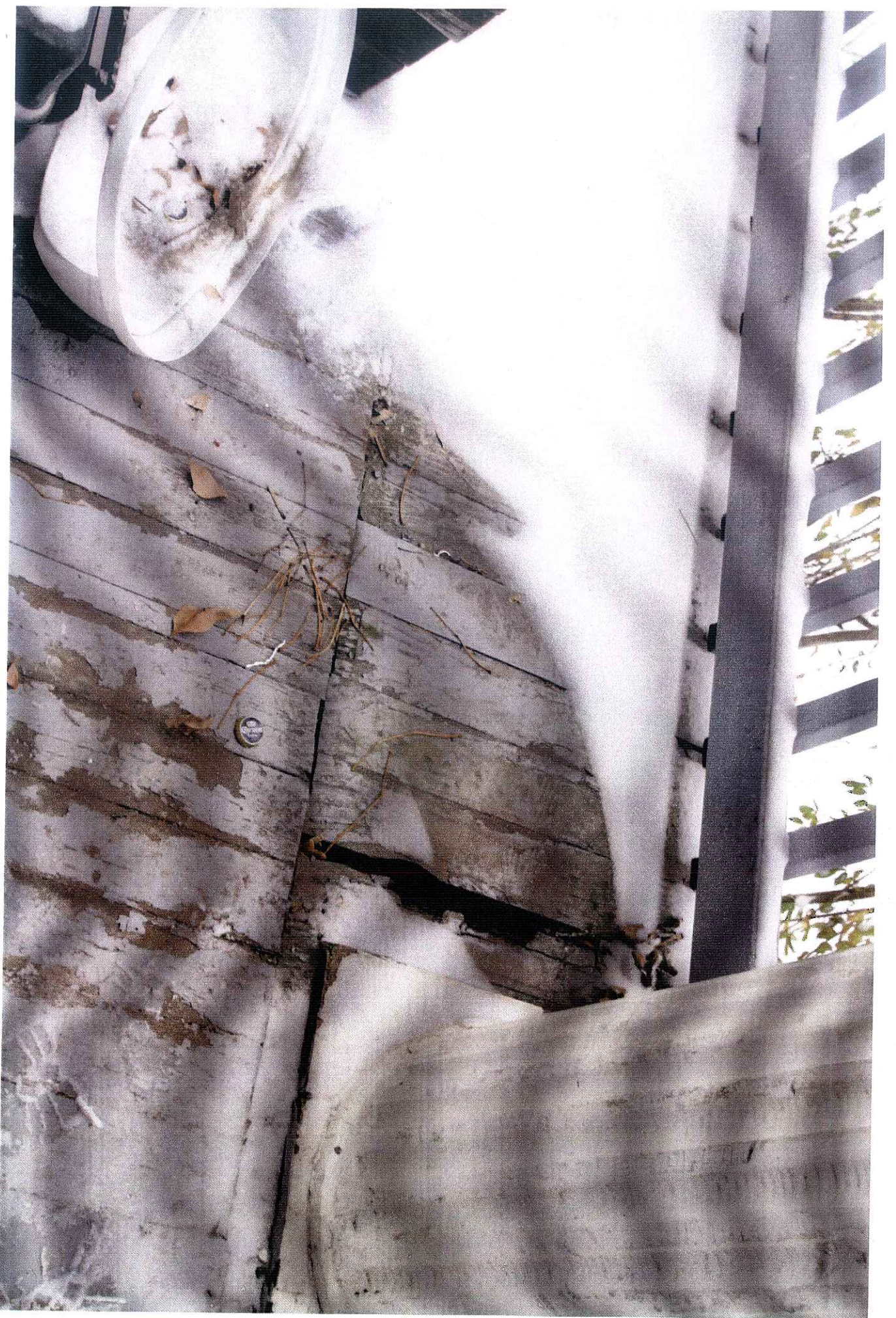
419 W. DAYTON - EXAMPLE OF ROTTING PATCHED PORCHES
