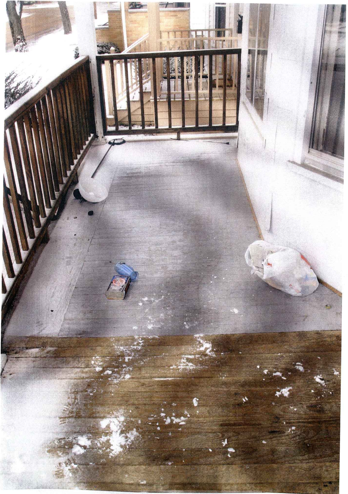
417 W. DAYTON – EXAMPLE OF ROTTING PATCHED PORCHES
