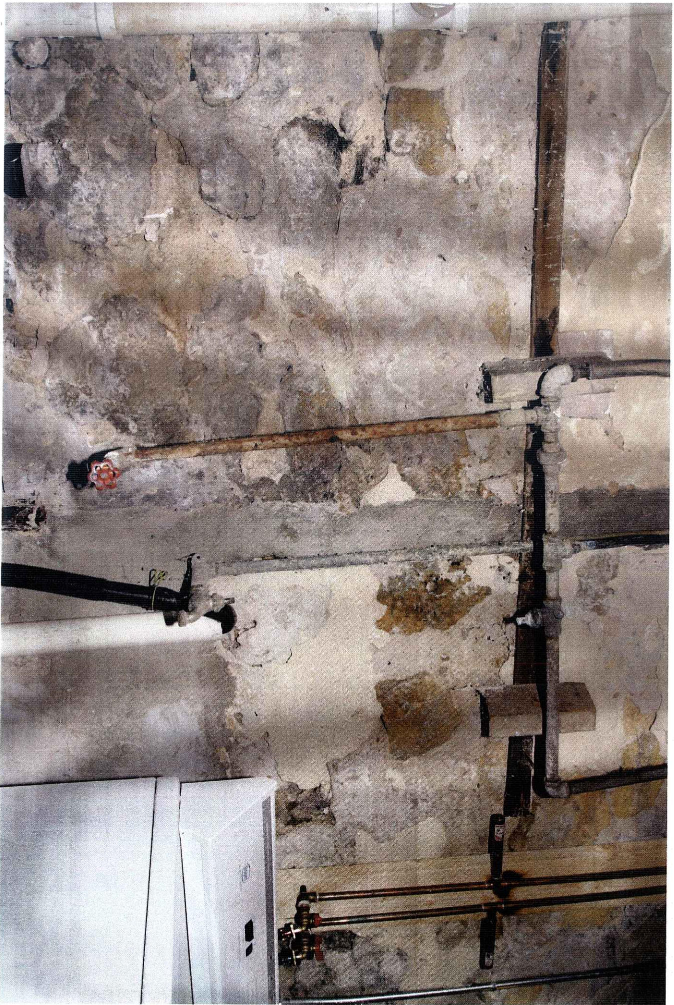
419 W. DAYTON - NOTE: LEAD, PVC, COPPER & GALVANIZED "COMBO" PLUMBING
