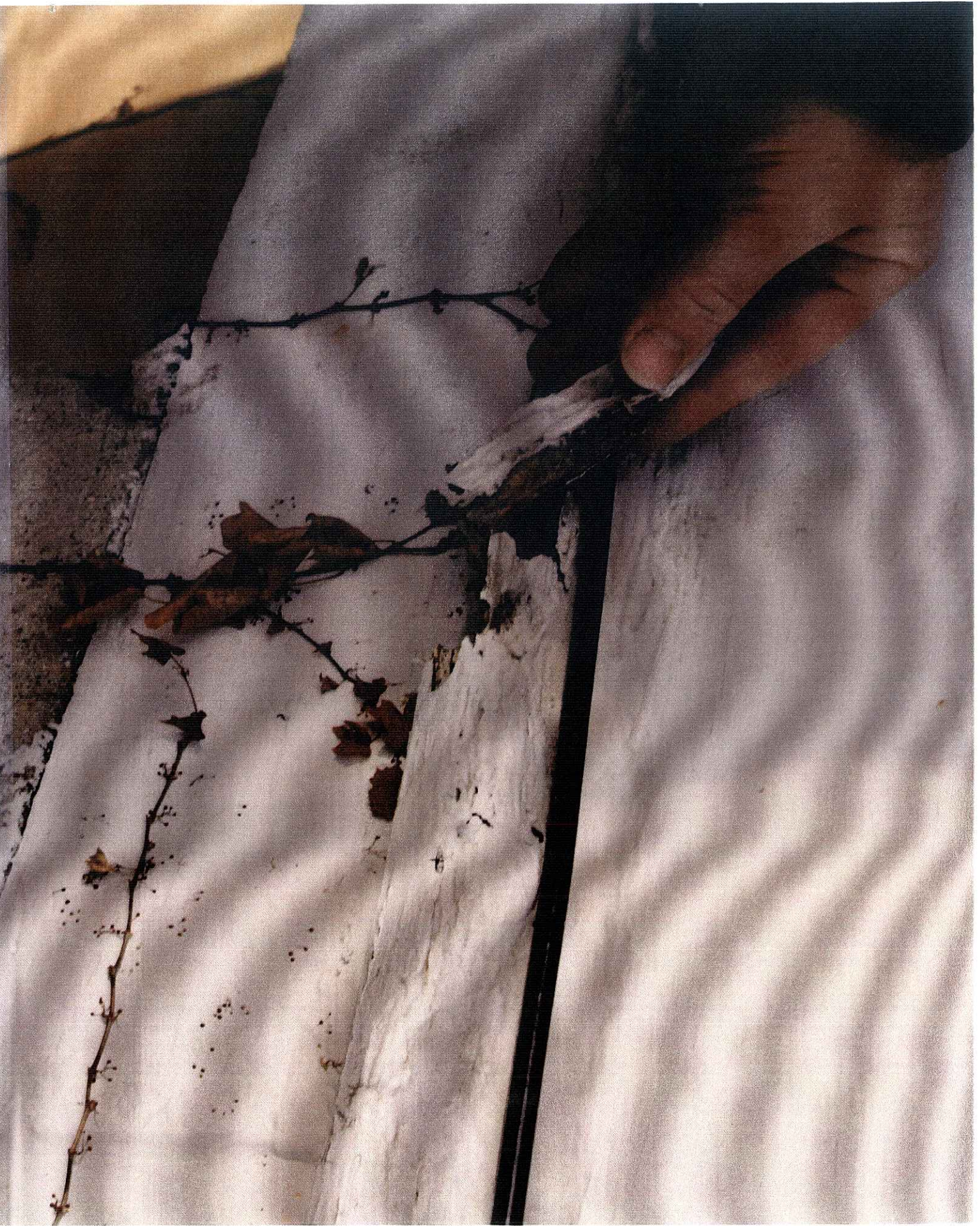
415 W. DAYTON - EXAMPLE OF ROTTED EXTERIOR WOOD THAT HAS BEEN PAINTED AND CAULKED OVER
