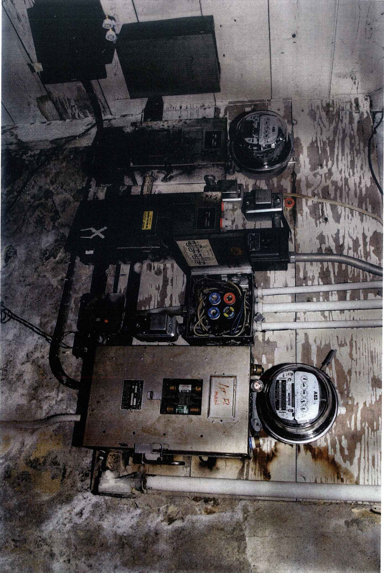
EXAMPLE OF INADEQUATE WIRING AND ADD-ONS
