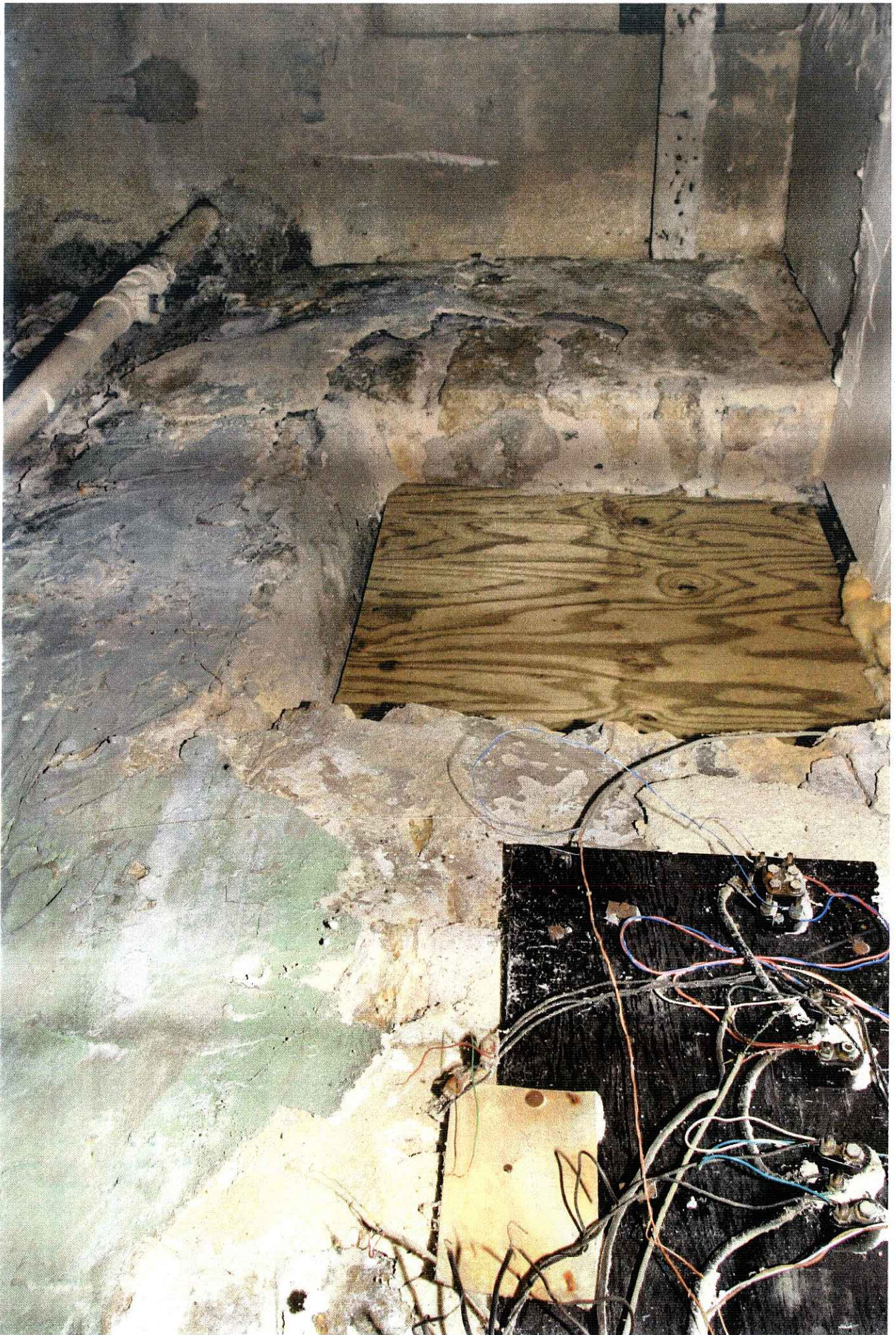
419 W. DAYTON - BASEMENT WALL. NOTE: SLOPING/PUSHED-IN WALL
