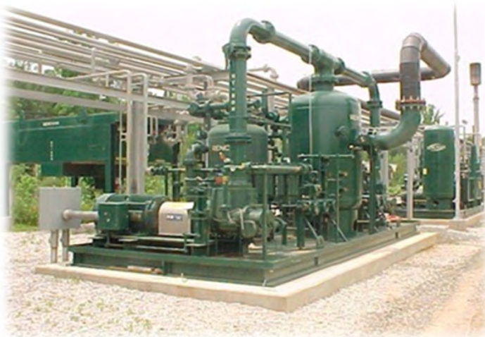
Biogas Compression, Upgrading & Injection
