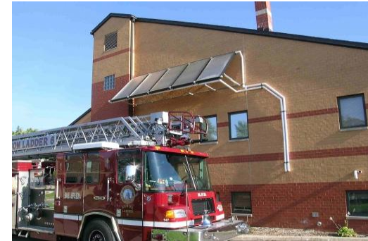
Solar hot water panels on Madison Fire Station 6 provide a good nonresidential example
