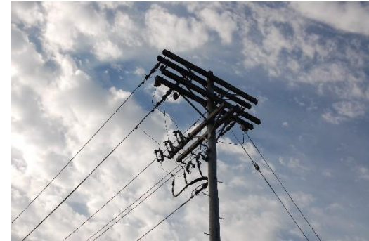
Existing overhead transmission lines on the north side of Cottage Grove Road
