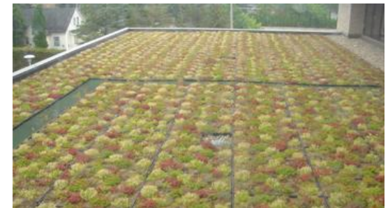
Green roofs can assist with stormwater management.
