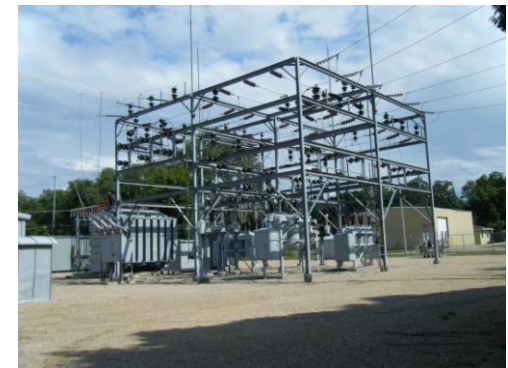
The MG&E Substation (above) will remain, but the buildings associated with the Royster-Clark fertilizer plant are no longer in use.
