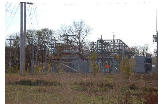
The MG&E Substation will remain on the site and may double in size in the long term
