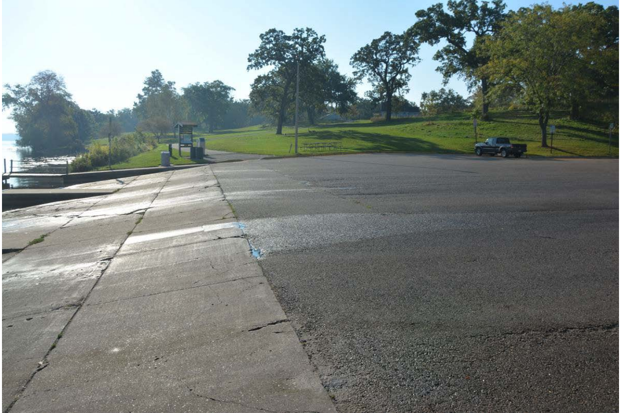
Existing condition of concrete at time of investigation. View to southeast.
