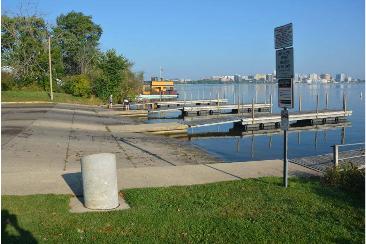
Existing condition of concrete at time of investigation. View to northwest.
