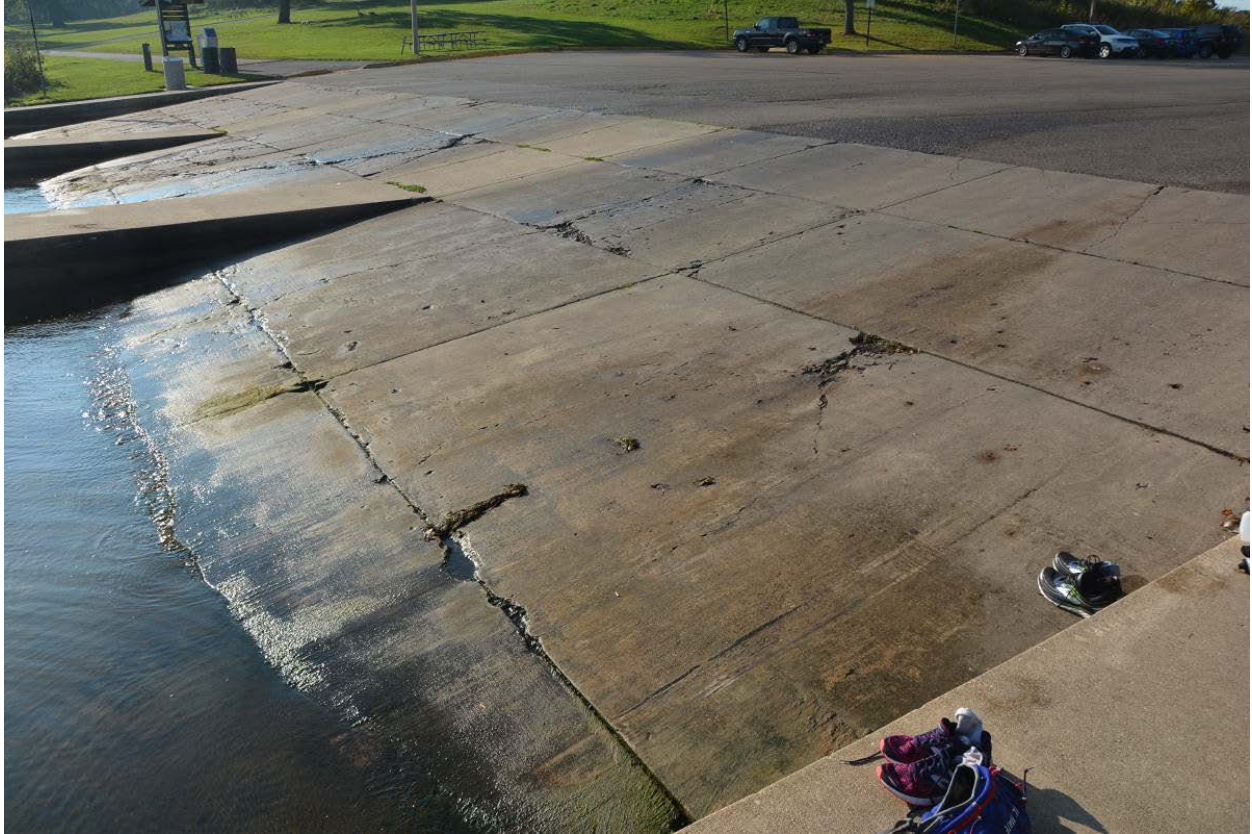
Existing condition of concrete at time of investigation. View to south.
