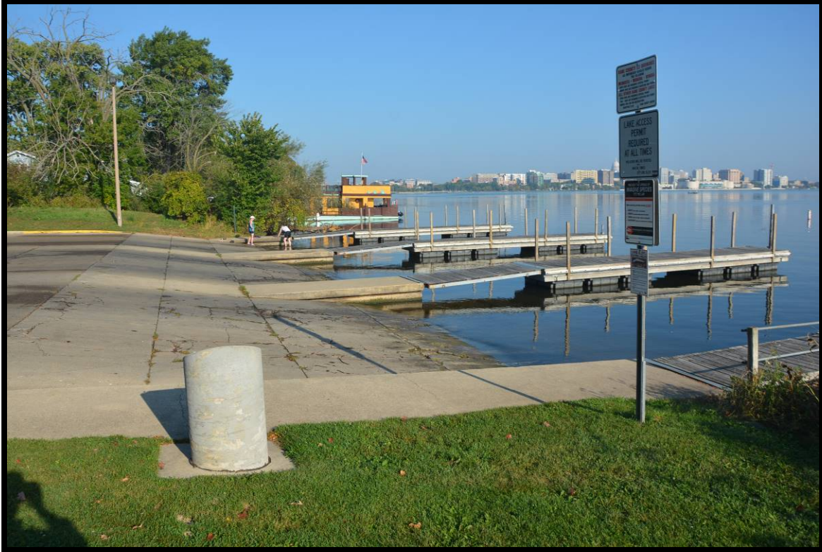
Figure Ten: Existing condition of concrete at time of investigation. View to northwest.
