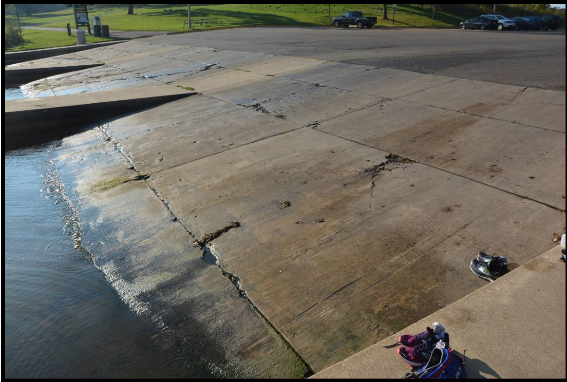
Figure Eight: Existing condition of concrete at time of investigation. View to south.
