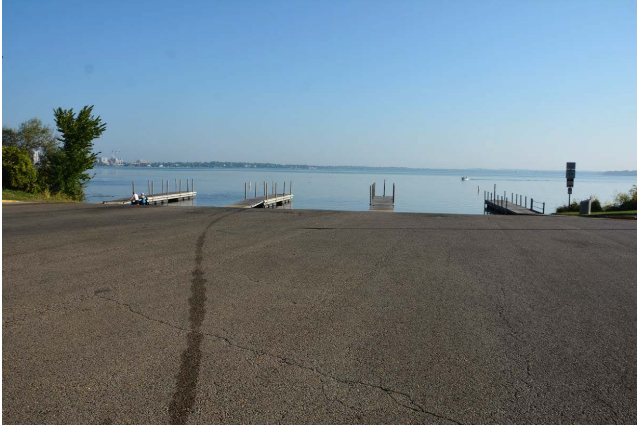
Existing condition of concrete at time of investigation. View to northeast.
