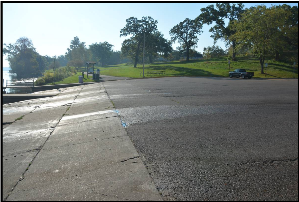
Figure Nine: Existing condition of concrete at time of investigation. View to southeast.
