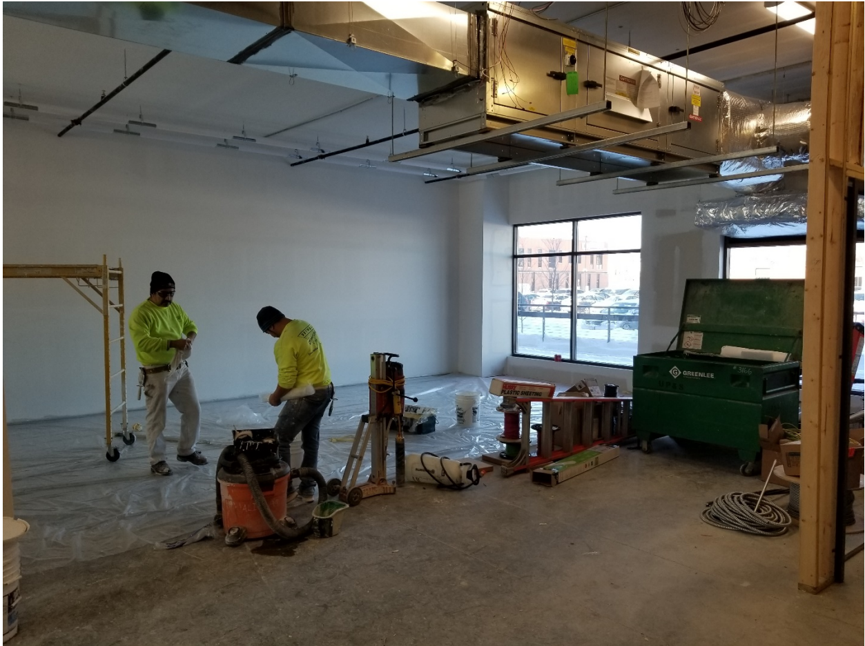
Back area being prepped for installation of 2 walkin coolers to be done on 2/15/19
