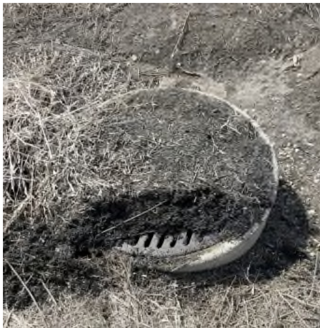
Figure 3-4: Infiltration Basin Outlet Structure clogged by Mulch and Dirt
