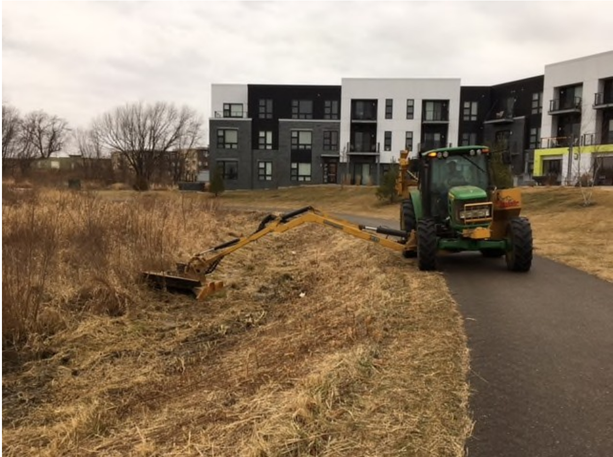
Figure 5-3. Public Works Crews use a Forestry Mower to remove Willows in a Swale near E Cheryl and Lacy
