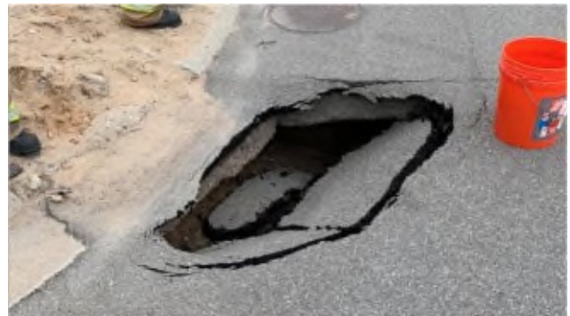
Figure 3-1: Sinkhole in Roadway
