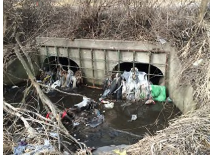
Figure 3-3: Outfall Partially clogged by Litter
