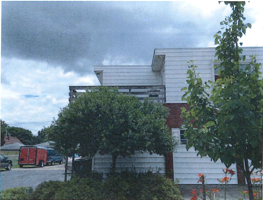
Vahlen façade-east. New siding, new railing, new lighting, and metal coping along edge where siding and brick meet.
