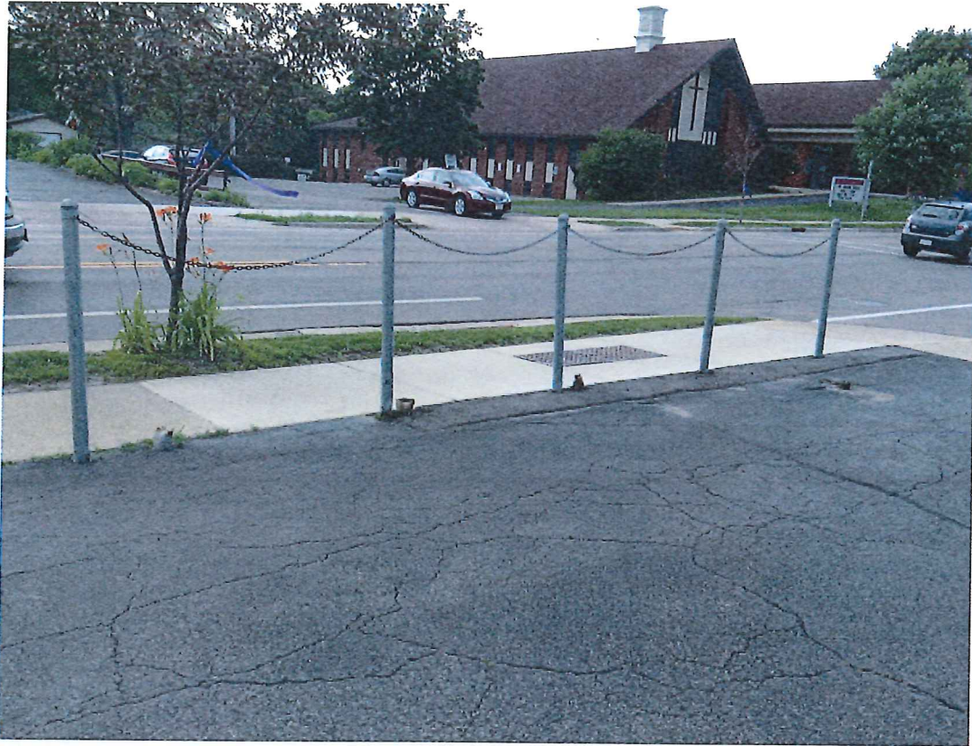
Parking lot facing west. Old posts to be cut out below grade.
