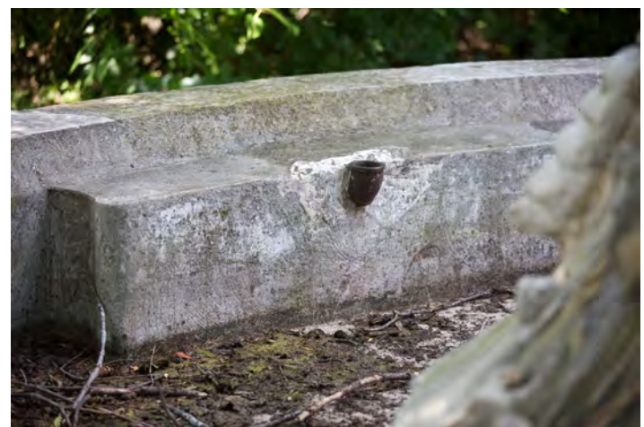
Figure 40: View of base of "wet" Triton
