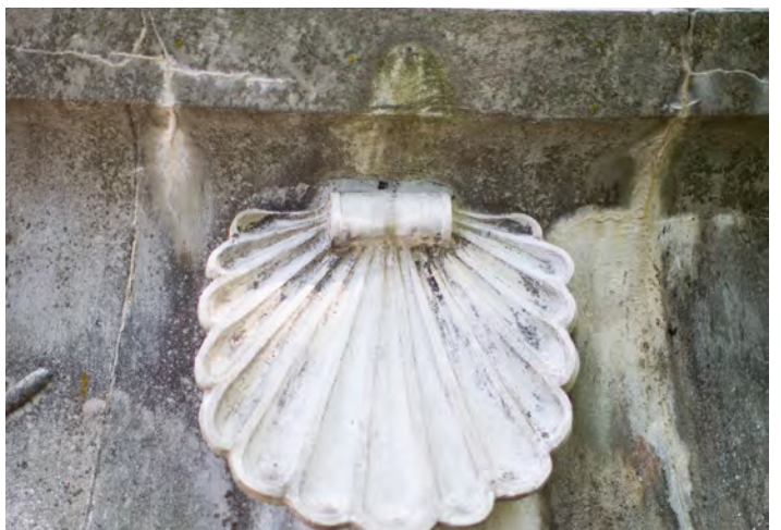
Figure 49: View of weep holes at shell, cracked limestone mineral deposits and trailing water
