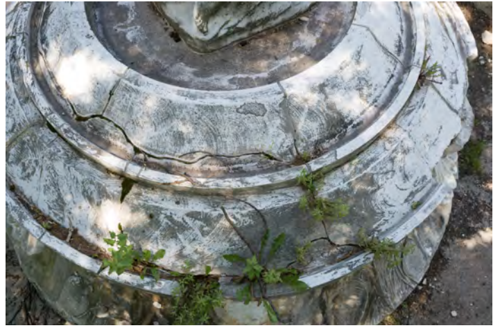
Figure 8: Upper view of pedestal and base - note damage to pedestal has been repaired and appears to have stabilized
