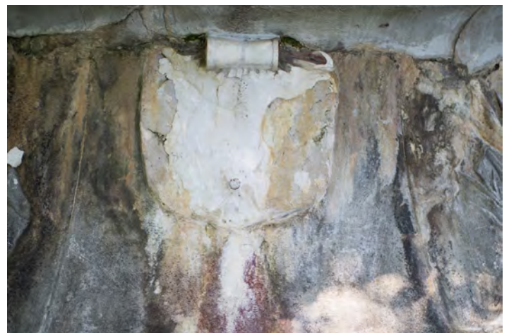
Figure 52: View of missing shell
