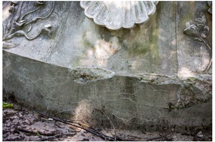
Figure 32: Degradation and mineral staining at trailing water
