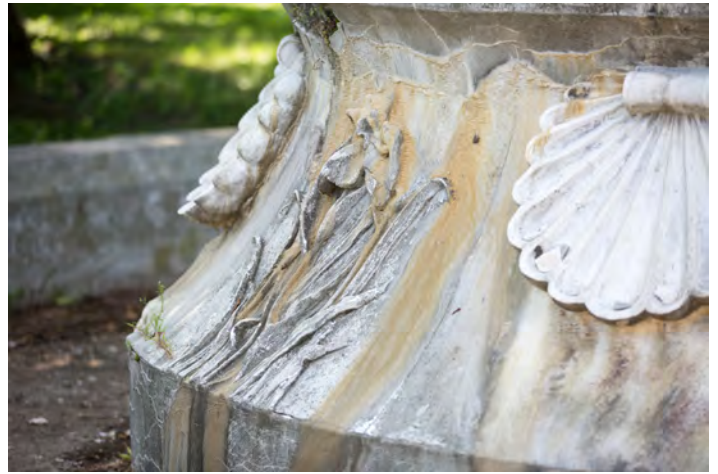
Figure 38: Shell motif condition amid mineral deposits at trailing water
