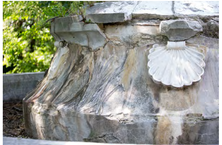
Figure 21: Excessive limestone damage adjacent to steel tension ring - causing iron oxide (rust) staining
