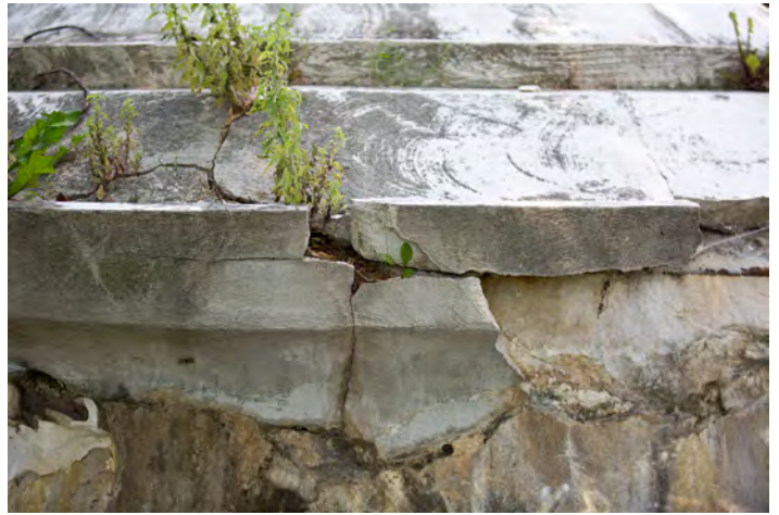
Figure 41: View of extreme damage to the limestone
