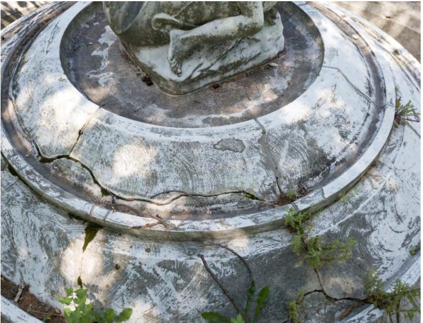
The transition from marble to limestone has fared poorly overall, but better than some of the “downslope” details. This is likely due to the fact that it was designed to handle significant amounts of water.
