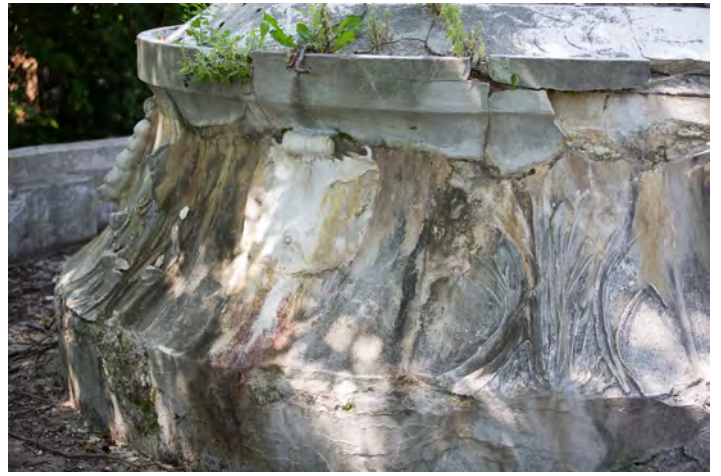
Figure 26: Excessive damage and improper repair with organic growth that is indicative of the level of disrepair
