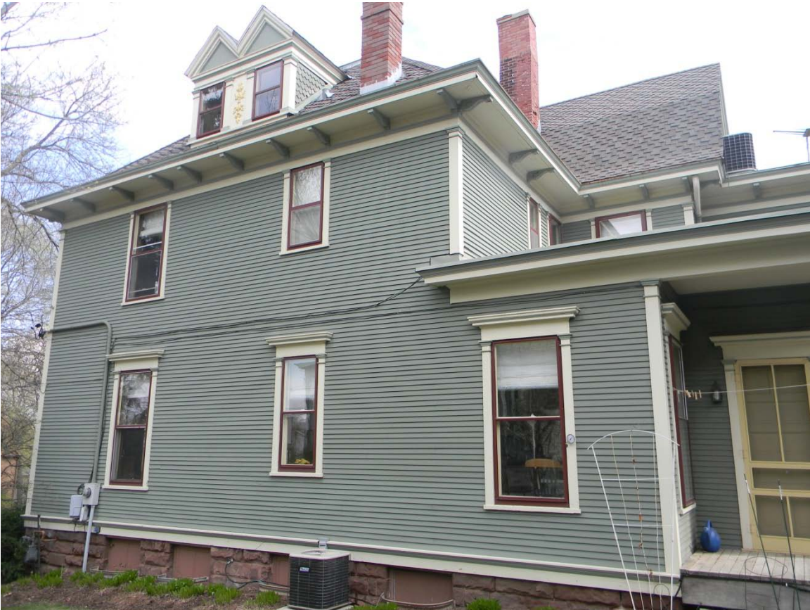
West façade: showing the first and second floor storms/screens to be replaced , and four basement windows to be filled-in with brick to match, with a 2-inch reveal.
