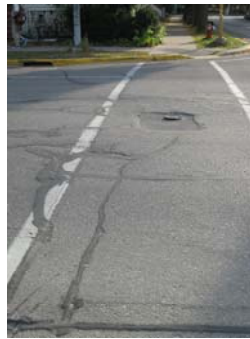
Basset-Dayton Crosswalk (cracks, tarred cracks, sinking patchwork)
