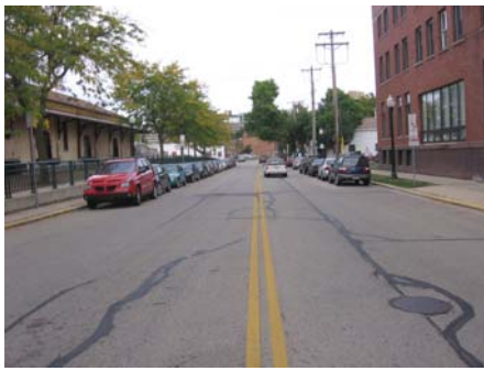
Bedford Looking NW (cracks, tarred cracks)
