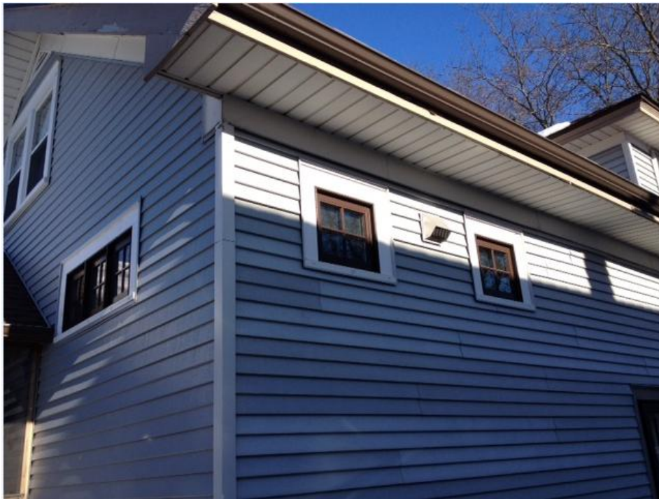
12. 1 st Floor Kitchen Windows – maintain existing Marvin replacement windows; replace siding with L.P. Smart Side 3” profile lap siding; replace aluminum soffit with wood beadboard soffit
