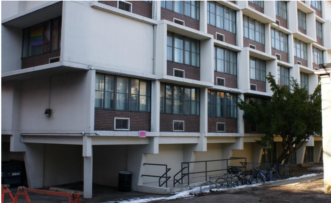
Master Hall East Elevation, Ground Floor Detail. Photo NW from SE by John Rolling 2/13/2026.
