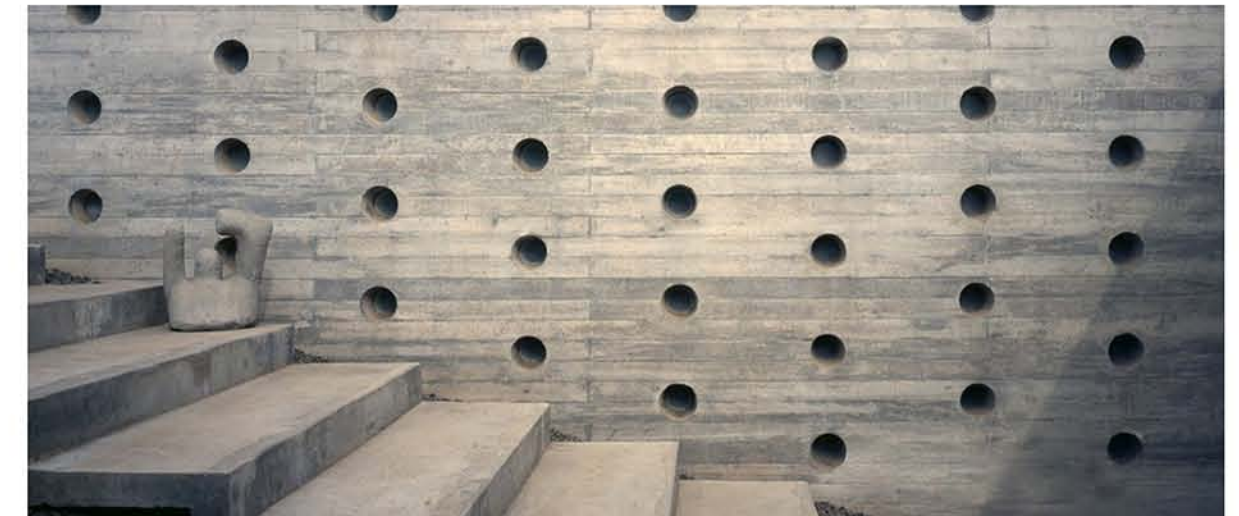
CONCRETE WALL HOLE FORM VOIDS interiii.com
