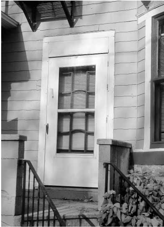
Storm door of insufficient height and inappropriate style
