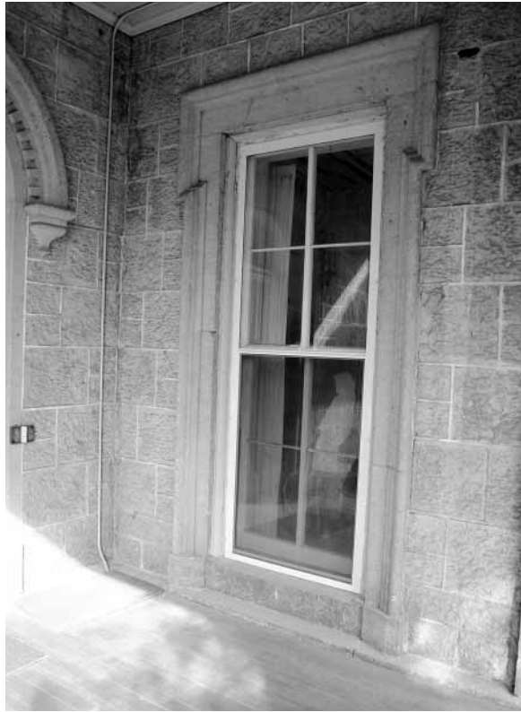
Same window as previous illustration with hand crafted replacement double hung window replicating original window. Photo by Ledell Zellars
