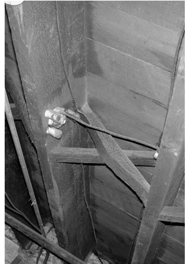
Many homes in Madison have knob-and-tube wiring still in active use.
