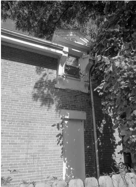
Inappropriate replacement window (top) that does not fill window opening resulting in partially covered window opening. Fully covered window opening (bottom).
