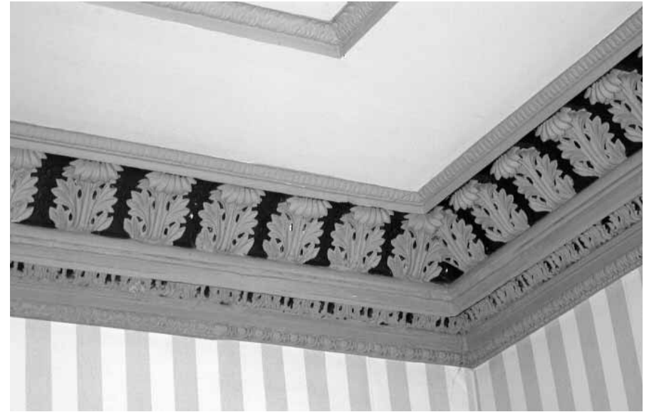
Ceiling detail in the McDonnell/Pierce House at 424 N. Pinckney St. Such features should be retained.
