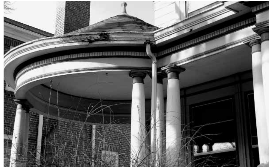
Poorly maintained roof
