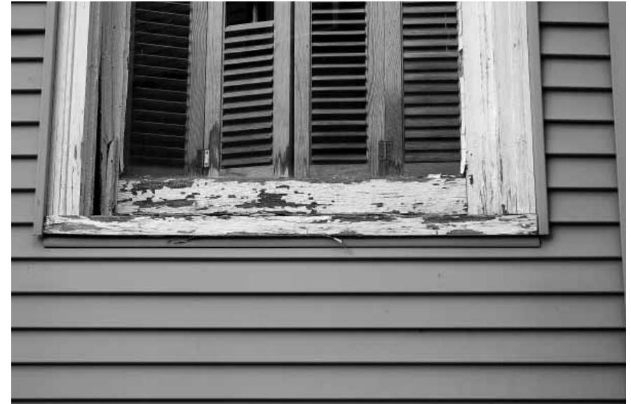
Window showing signs of deterioration and rot.
