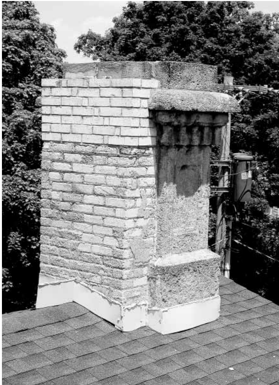
Chimney that has been "remuddled".
