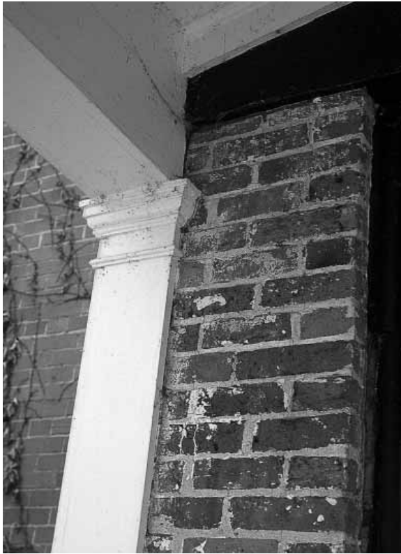
Poorly tuck-pointed brick
