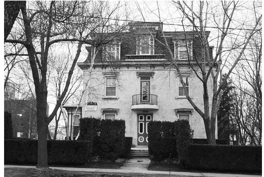
Kendall House 104 E. Gilman St. today having lost its porches and much of its architectural detail.
