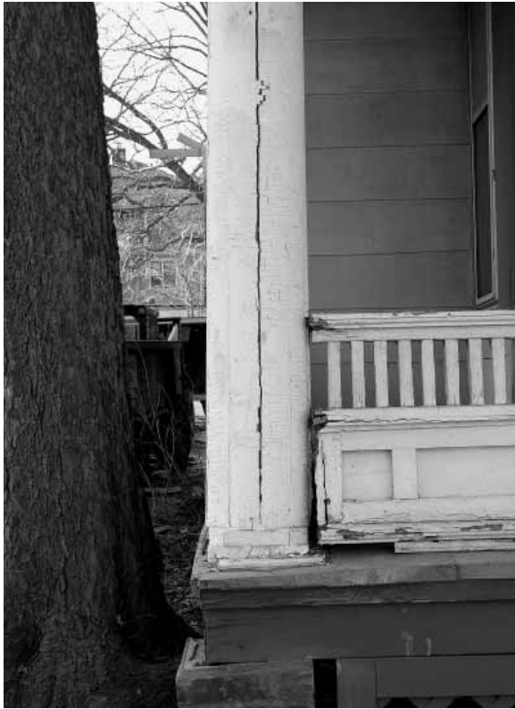
Deteriorating original 19th century porch. Photo by Ledell Zellers
