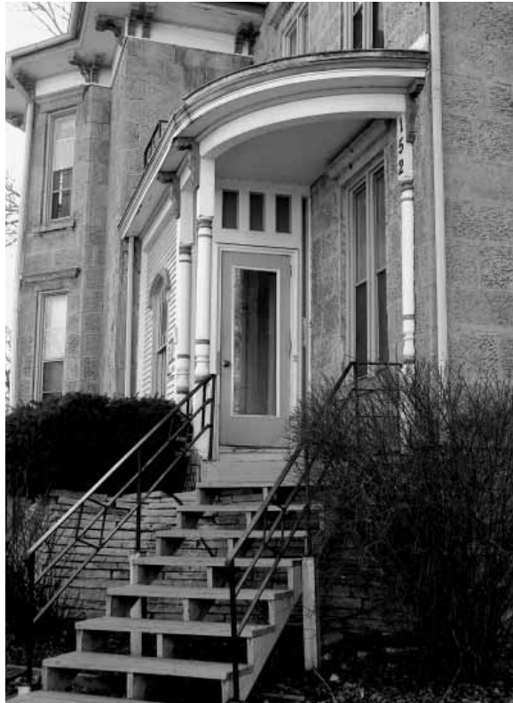
Inappropriate steps with open risers and out-of-character railings
