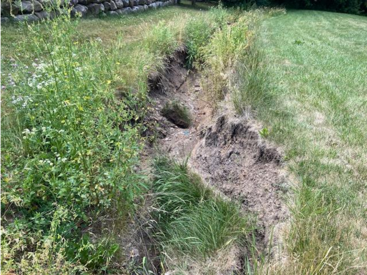
Upstream Channel Erosion – Just Downstream of Culverts
