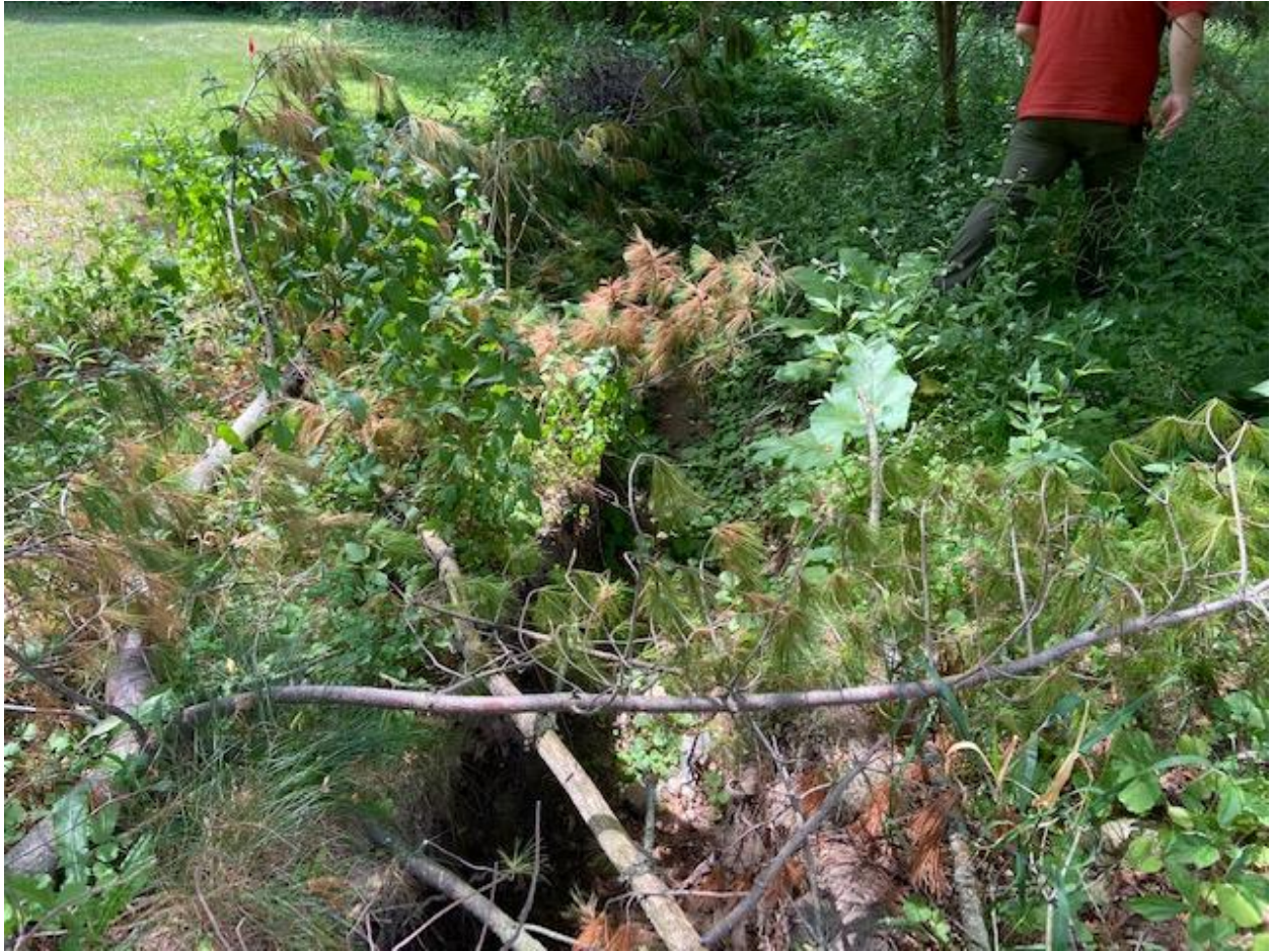
Channel Erosion – Just Prior to Basin Area
