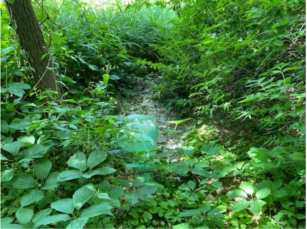
Outflow Pipe From Detention Basin
