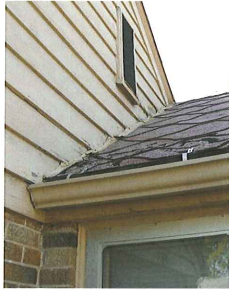
Deterioration of caulking and missing flashing at front porch roof interface with exterior wall
