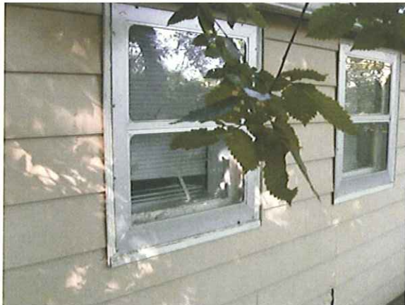
Broken/non-operable single pane window and storm
