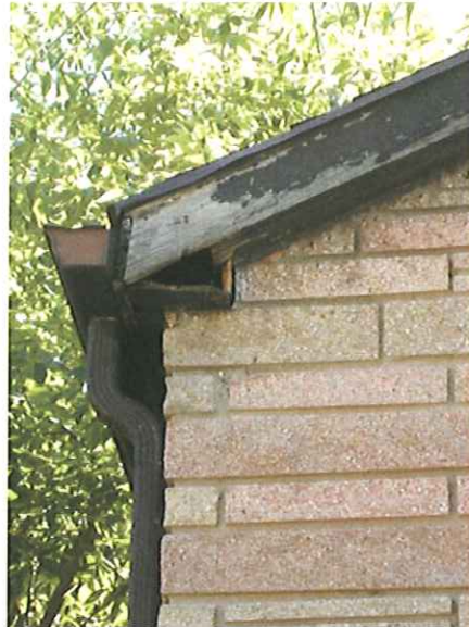
Rot and noticeable openings in eaves
