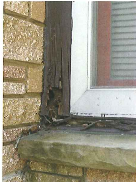
Rot and insect damage at wood window trim
