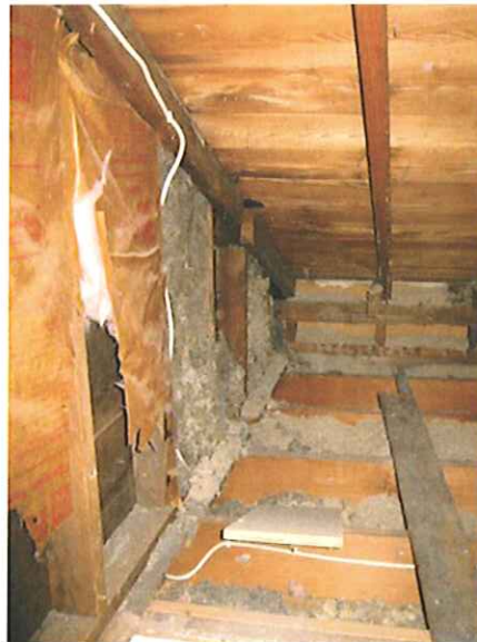
Limited insulation/chewed insulation within the attic
