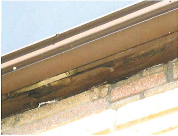
Rot at wood eave/masonry interface
