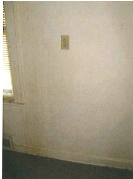
Water staining on wall around window
