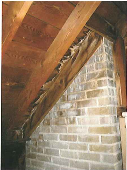
Water staining on roof sheathing and masonry at chimney
