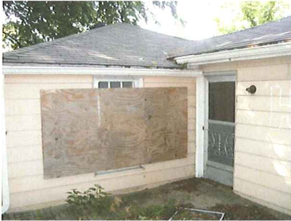
Damage to metal siding and detail of siding continuing below grade
