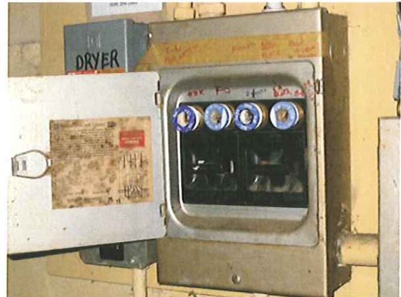
Outdated electrical system (no ground at the outlets)
