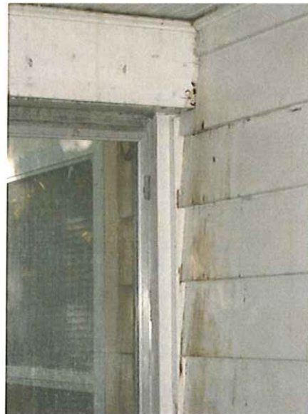
Water staining at back porch
