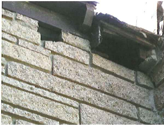
Rot and noticeable openings in eaves
