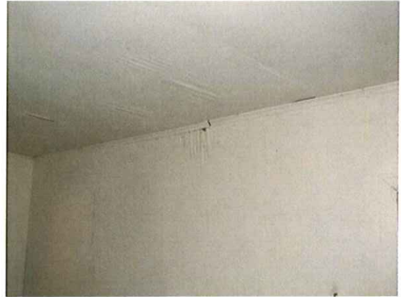
Water damage on ceiling and wall within bedroom
