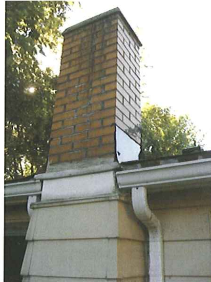
Water staining and attempts to correct at masonry chimney and metal siding interface
