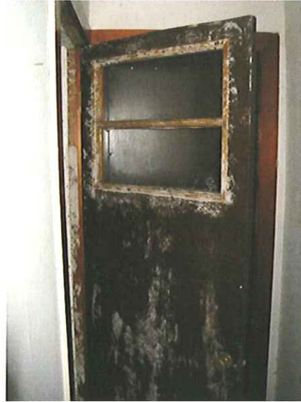
Mold on door leading to basement
