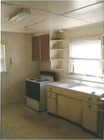
Sagging ceiling and water damage in kitchen ceiling/water on the floor
