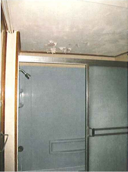
Peeling paint on bathroom ceiling
