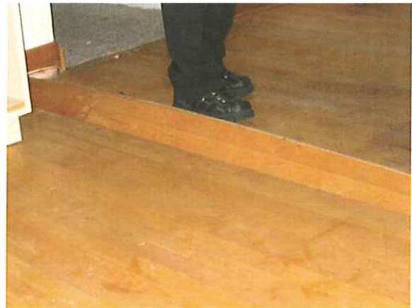
Swollen hardwood floors in main room
