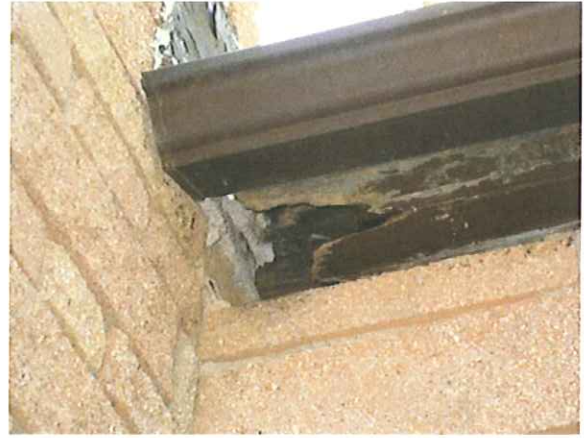
Rot at wood eave/masonry interface
