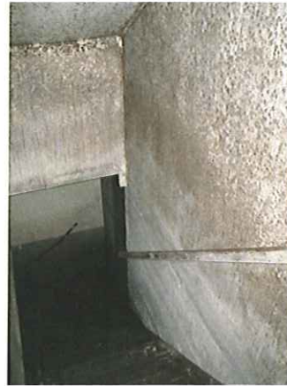
Mold throughout walls leading down to basement/water filled basement
