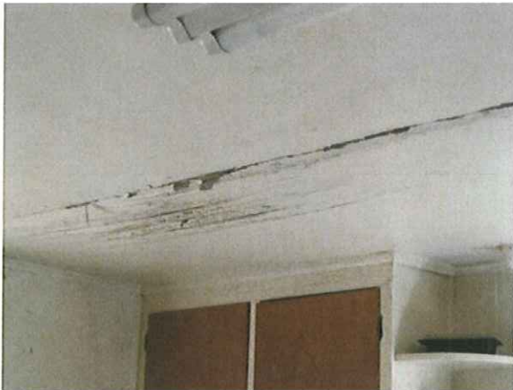
Water damage in kitchen ceiling
