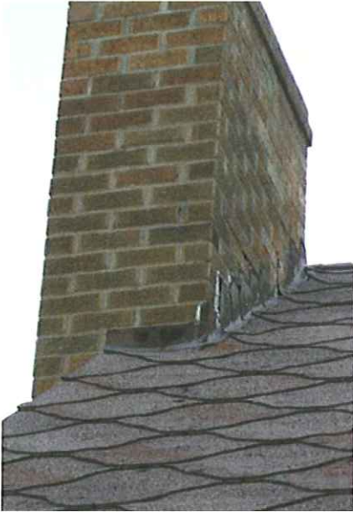
Caulk failing between flashing and masonry and flashing and asphalt shingles
