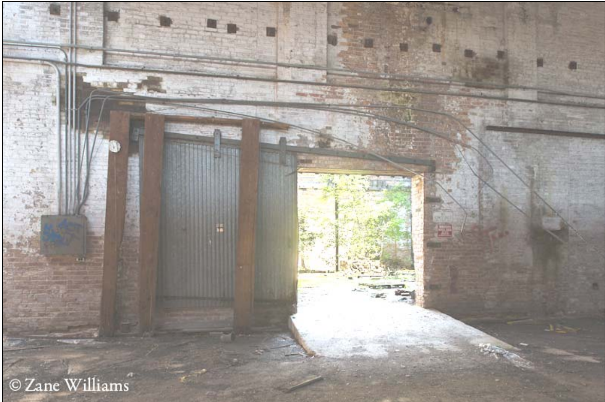
Image 28: Interior of main interior mill space, looking north to former feed storage area.
