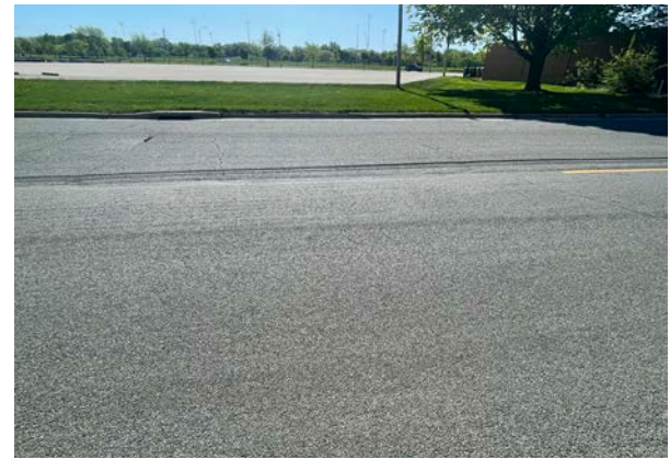
Pennsylvania Avenue (cracking, curb crumbling, some settling)
