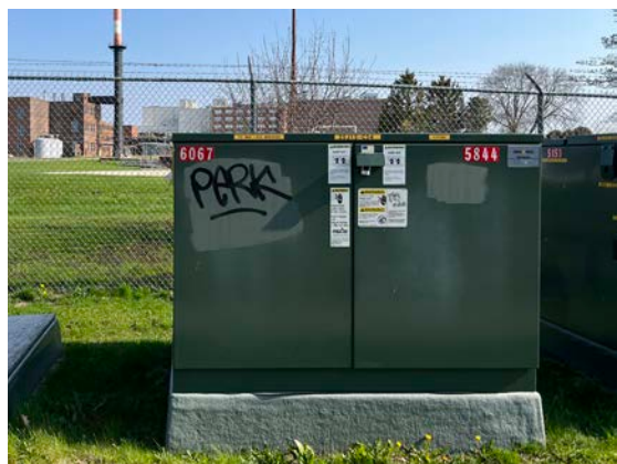
Commercial Avenue (graffiti on electrical box)
