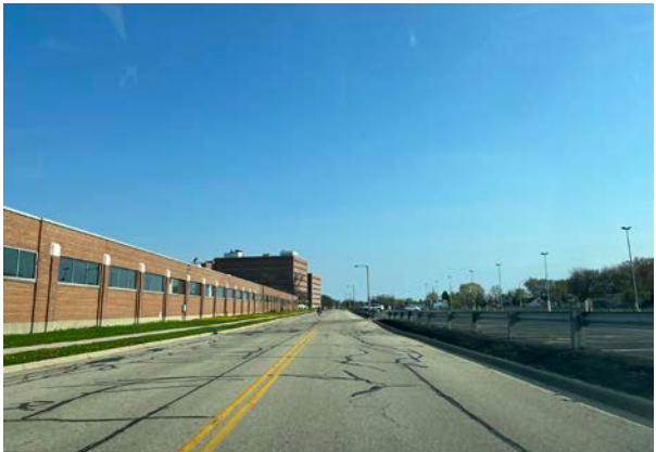
Oscar Avenue (tarred cracks, crumbling along gutters, fading center line paint)
