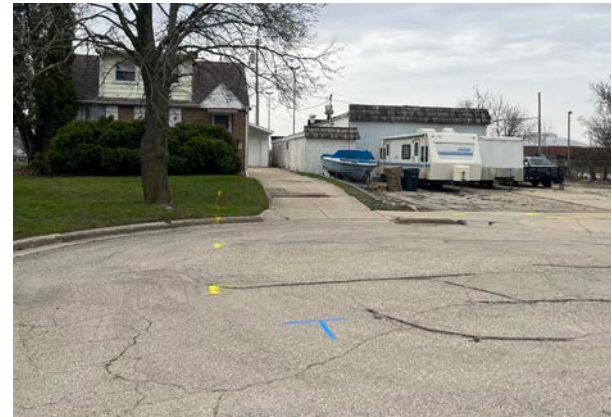
Myrtle Street (cracking, crumbling curb, aggregate showing)
