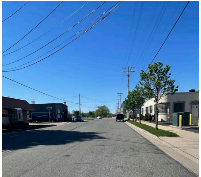
Pennsylvania Avenue (center line completely faded, chipping)
