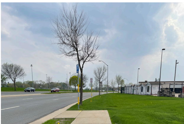
Packers Avenue (some cracking, otherwise good condition)
