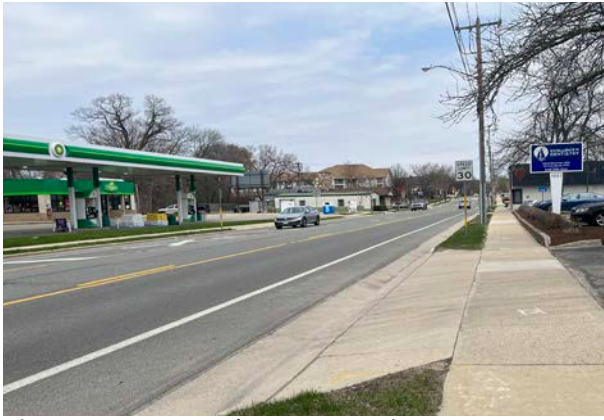
Sherman Avenue (aggregate showing, crumbling along gutter)
