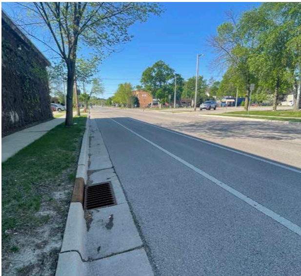
Fordem Avenue (some debris in gutter)
