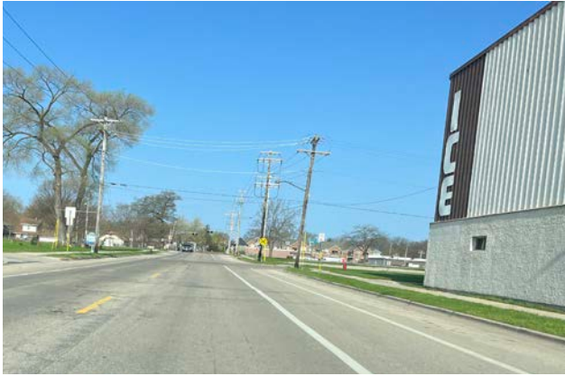
Commercial Ave (cracking, crumbling, some settling)
