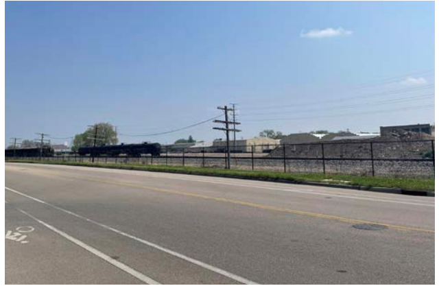
Fordem Avenue paint marks fading, generally good condition)
