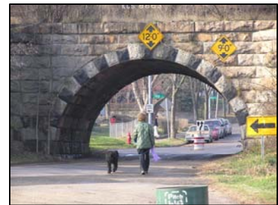
The railroad viaduct at Bram-Koster poses unsafe conditions for pedestrians because of its narrow width.
