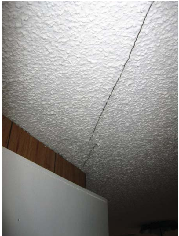
Photo 13 – Ceiling finish distress beneath roof
