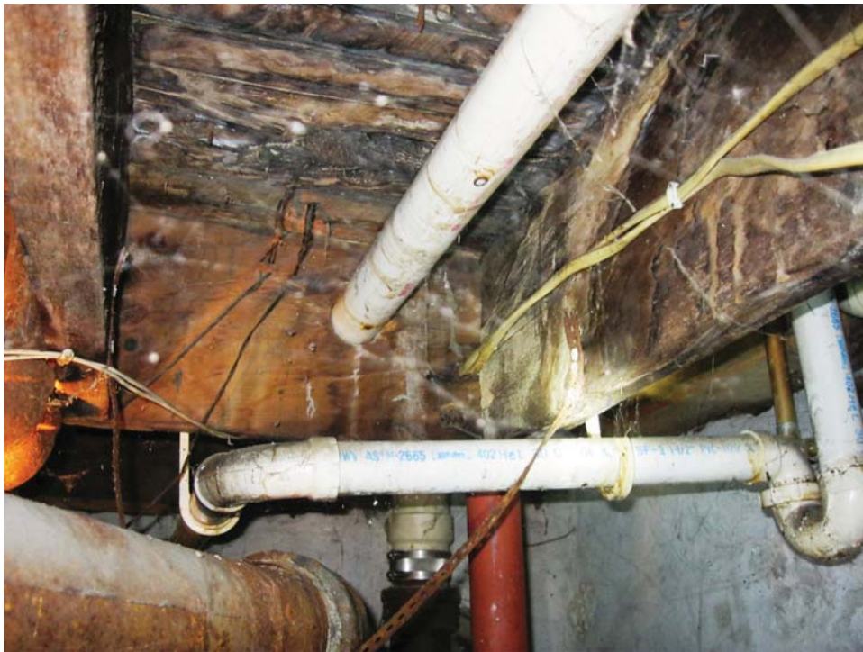
Photo 7 – 1 st floor framing with water damage
