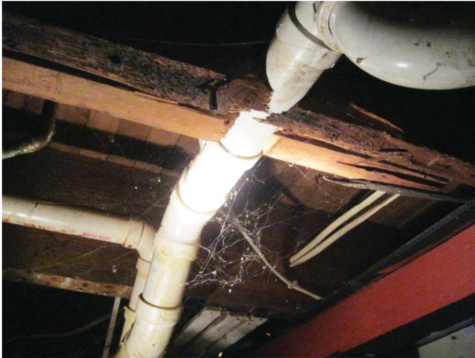
Photo 8 – 1 st floor framing notched for plumbing
