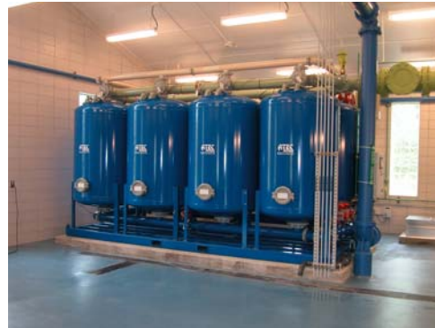
Iron and Manganese Filter at Well 29
