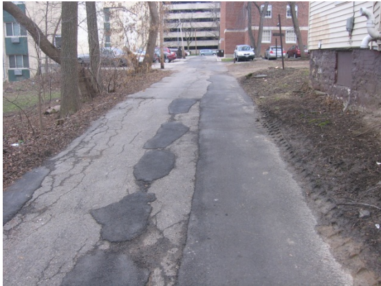
Asphalt problems in Sections B Alley (poor condition)
