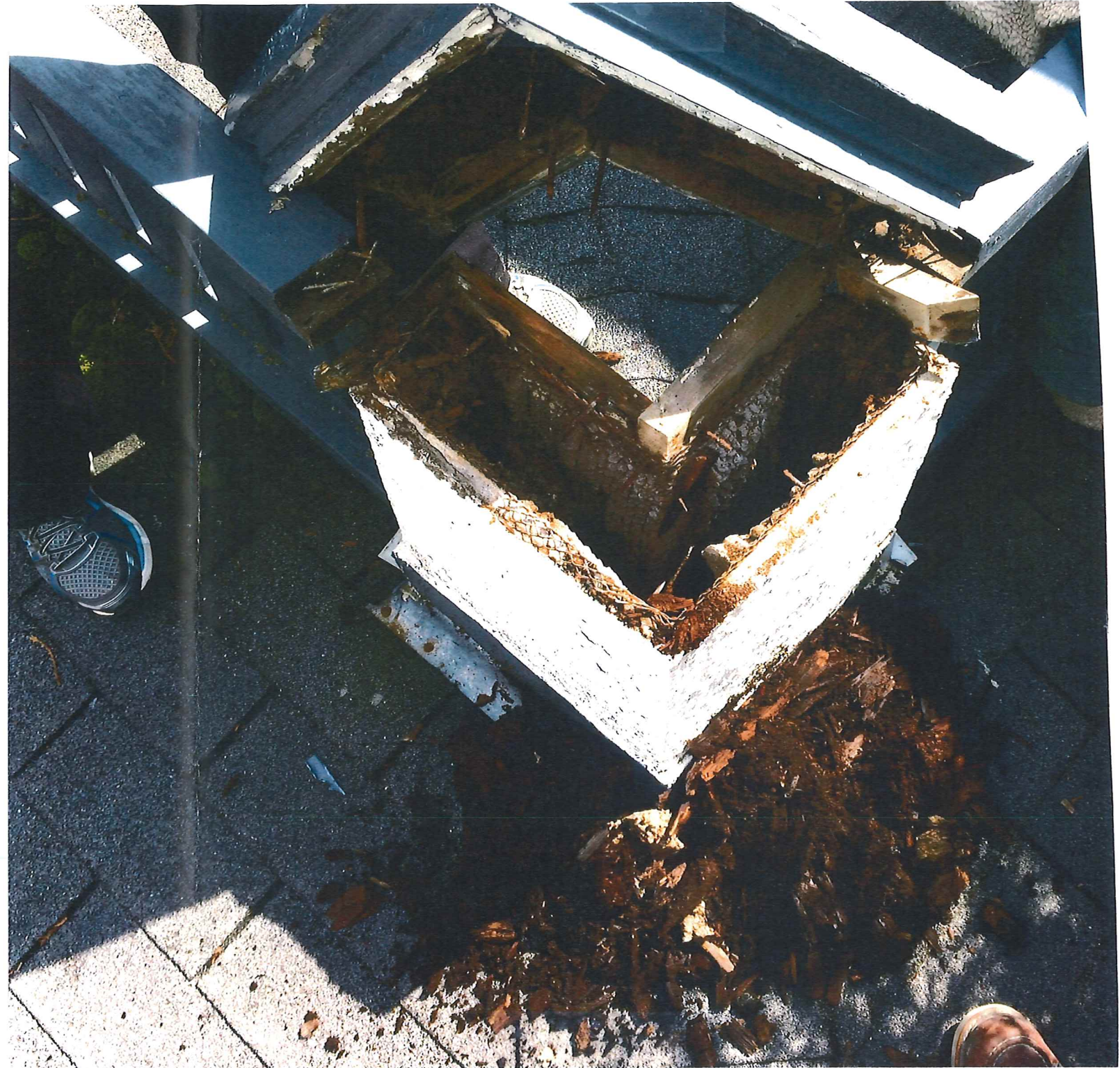
Interior Structure of Parapet has completely failed
